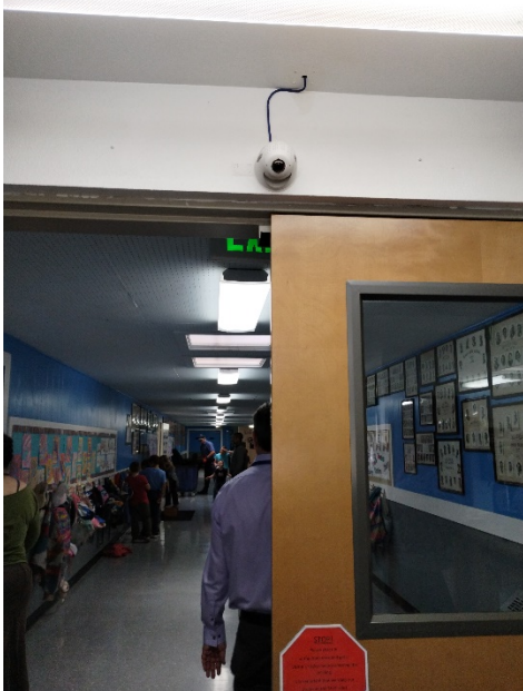
Prominent video security system. Cameras are a significant deterrent to unwanted behavior and vital for law enforcement.
