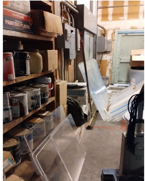
Facilities storage. Ensure minimum 33in of clear space around electrical panels.
