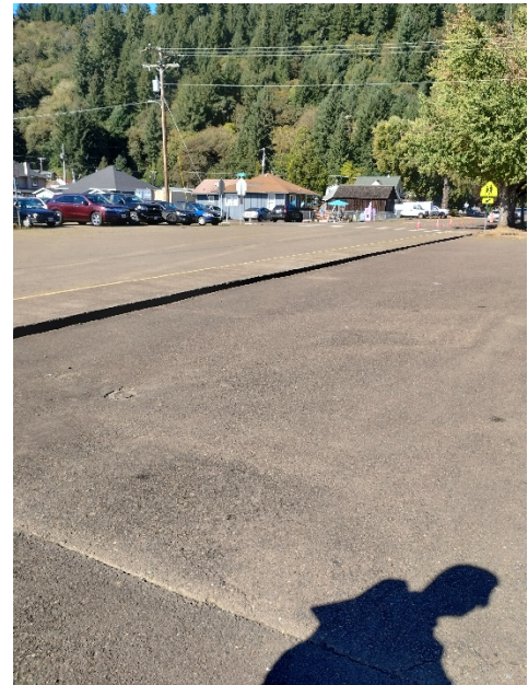
Student drop off and pick up area. Improve demarcation of pedestrian and vehicular pathways. Install barriers to protect pedestrian areas from vehicles.
