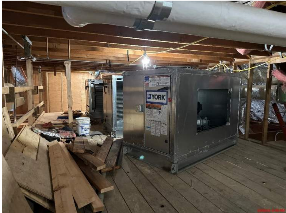
CHHS – air handler units in attic space
