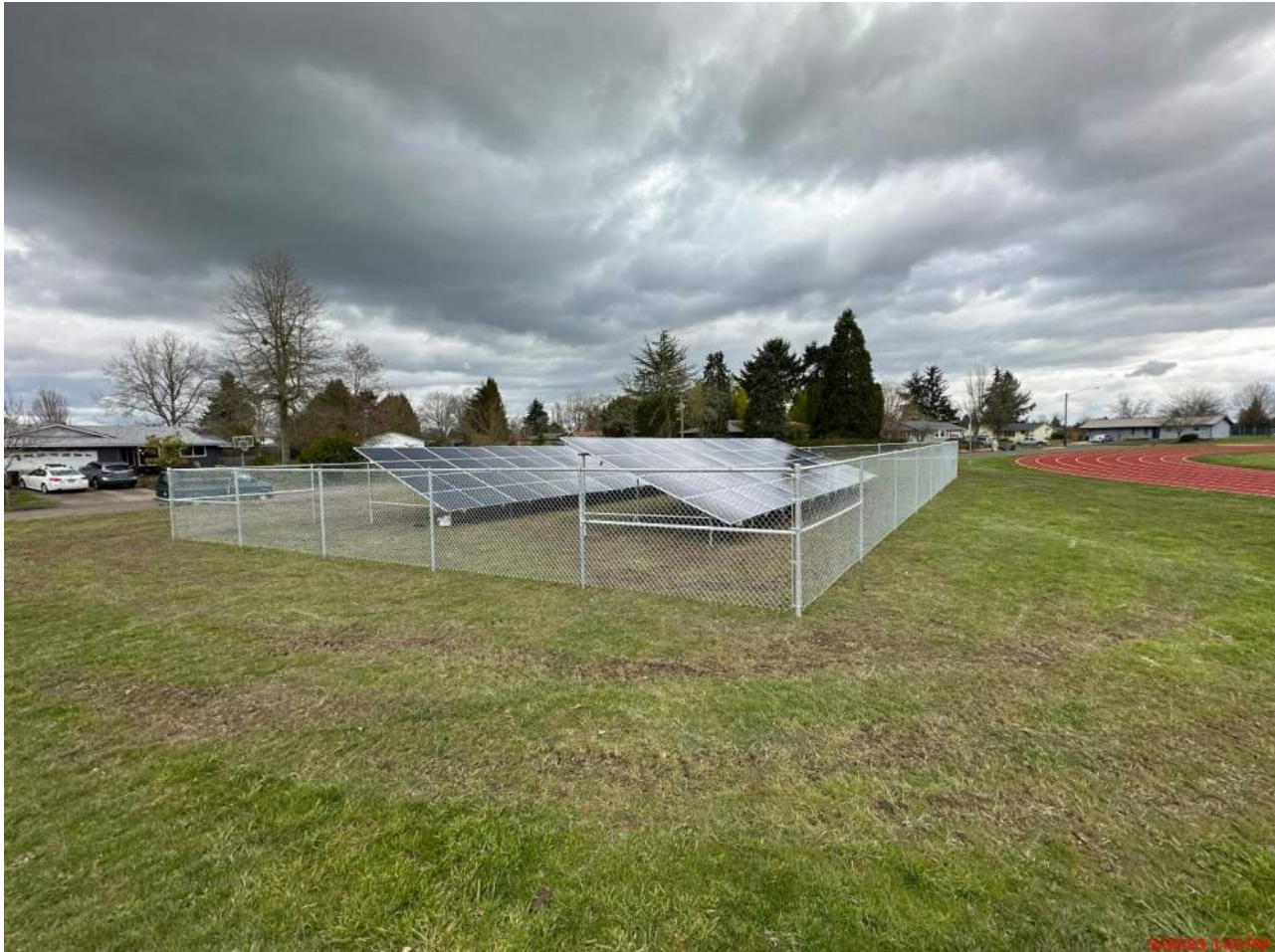
Cheldelin – New solar installation
