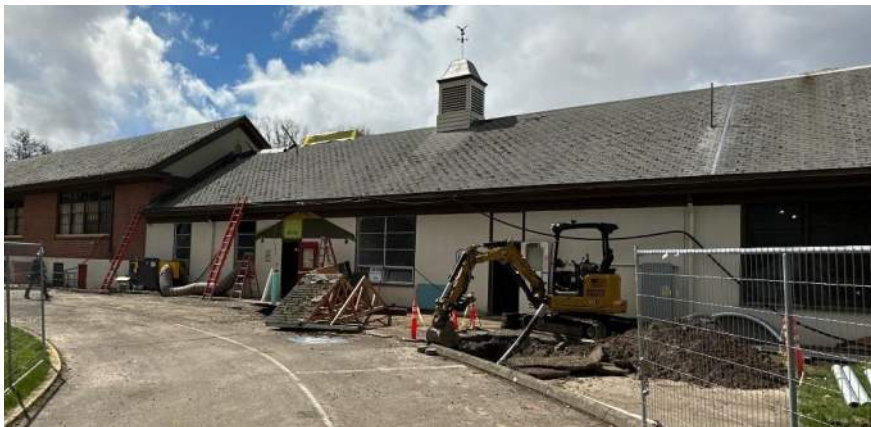
CHHS – Front entry canopy removed for new installation. (old canopy sitting in foreground)
