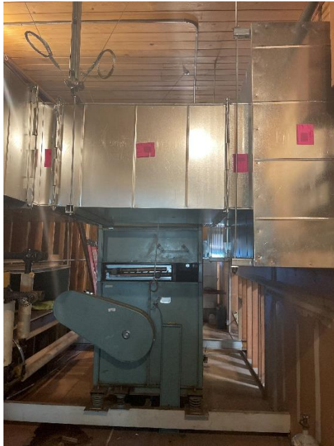
CMS – Refurbished Units and New Ductwork
