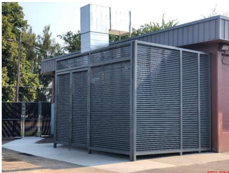
Dust Collector Screen Wall - current configuration
