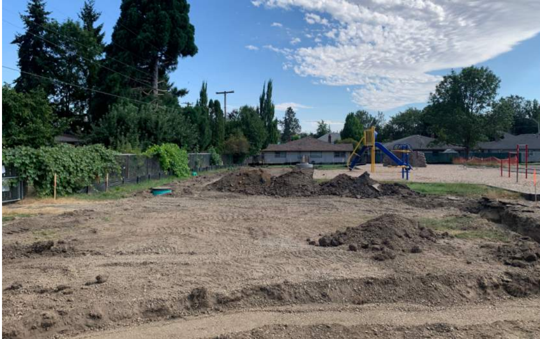
Storm detention system
