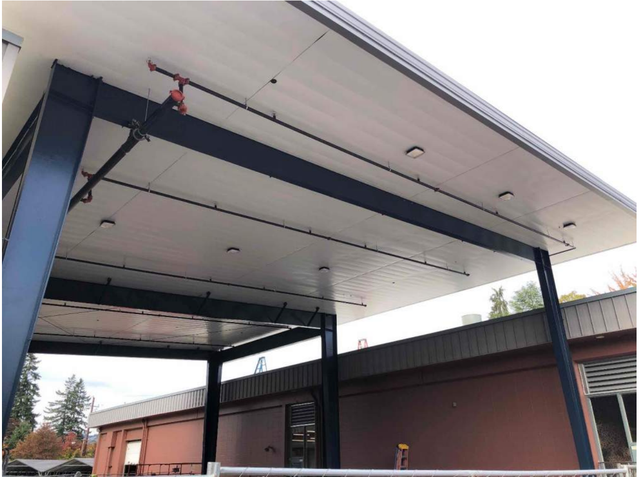
CHS – New outdoor covered work area soffit in place and finish painting wrapping up
