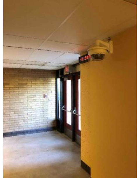
CVHS Building A & F – Typical camera and reader board installation
