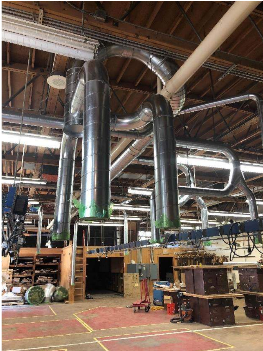
CHS – new woods dust collector piping
