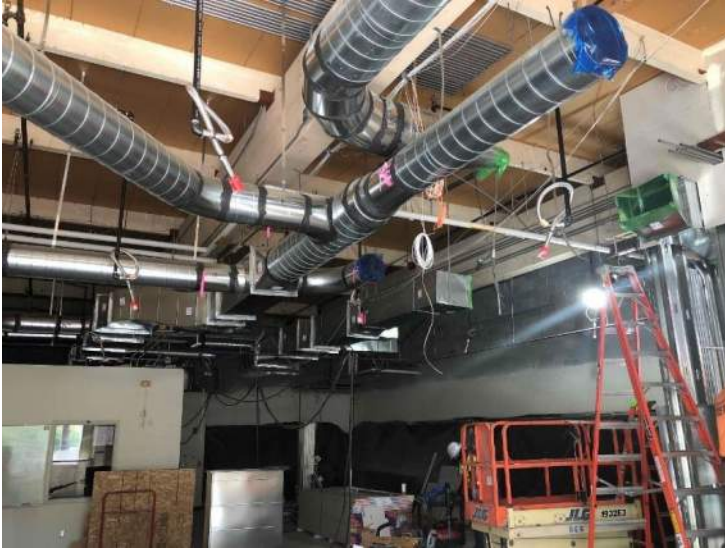
CVHS – new HVAC in ceramics ceiling
