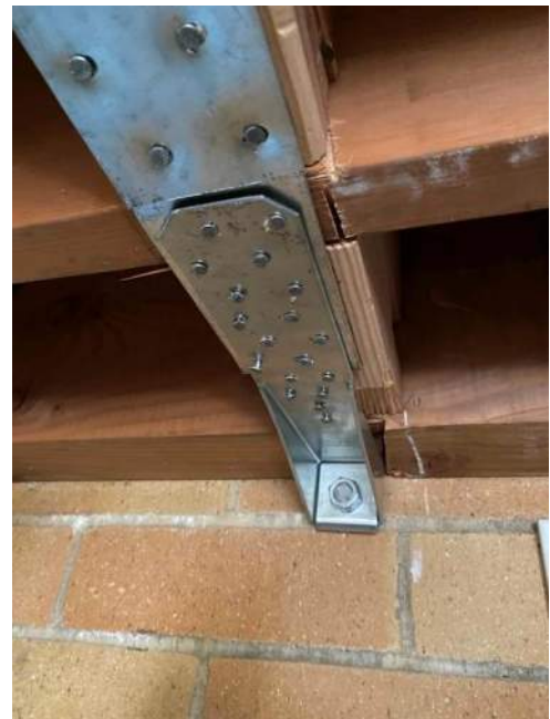
Library seismic strapping
