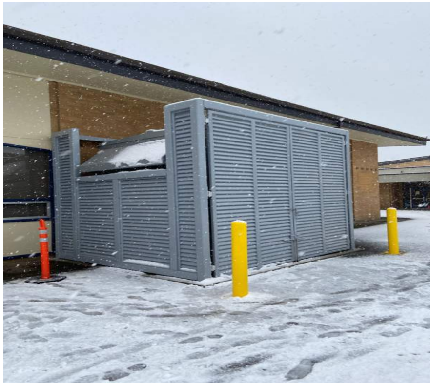
New HVAC enclosure outside STEAM
