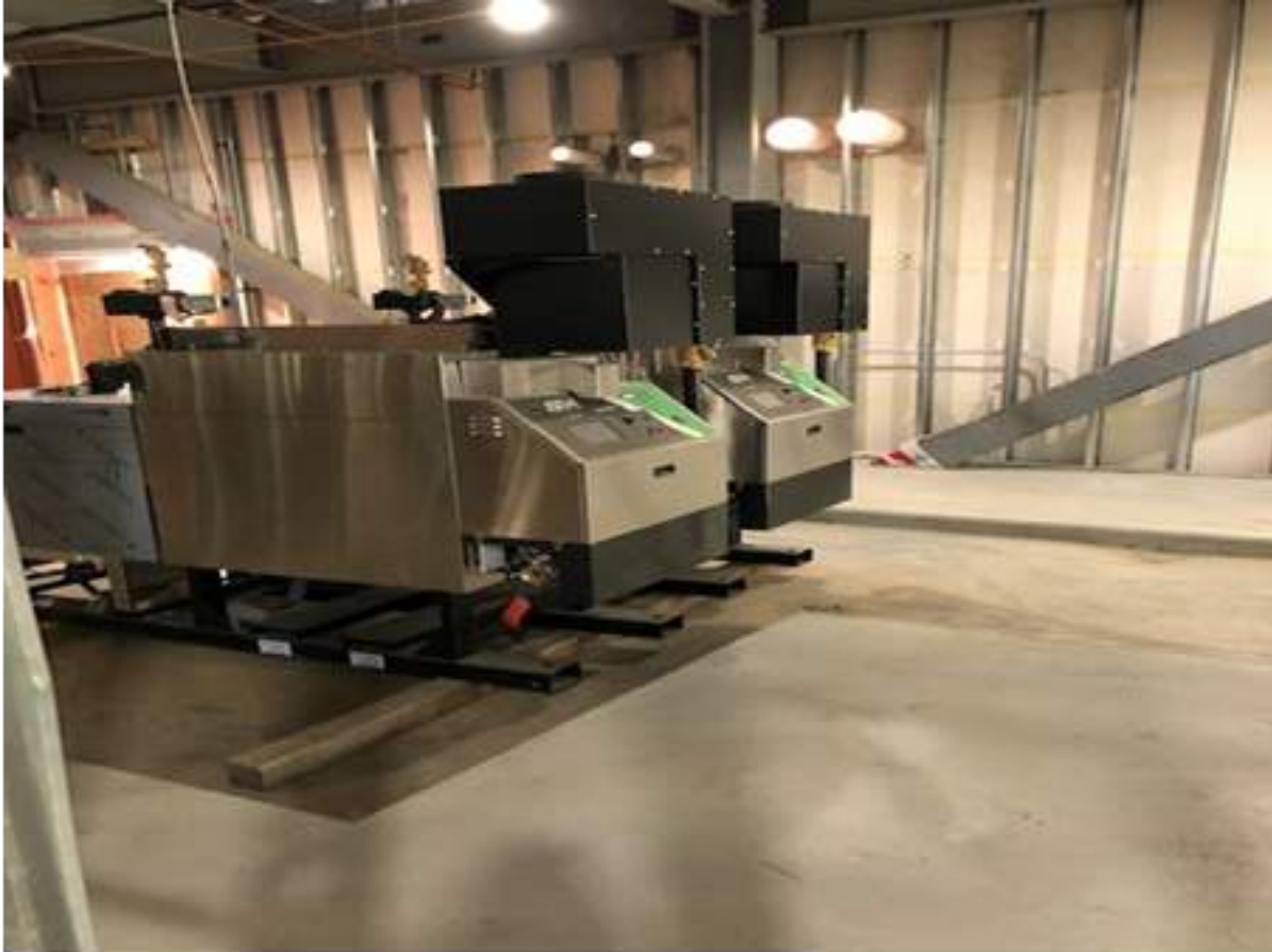
Mechanical equipment awaiting installation
