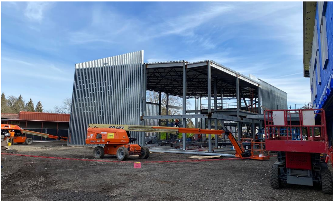
The Lincoln gym is rapidly taking shape with the very tall metal stud framing almost complete.
