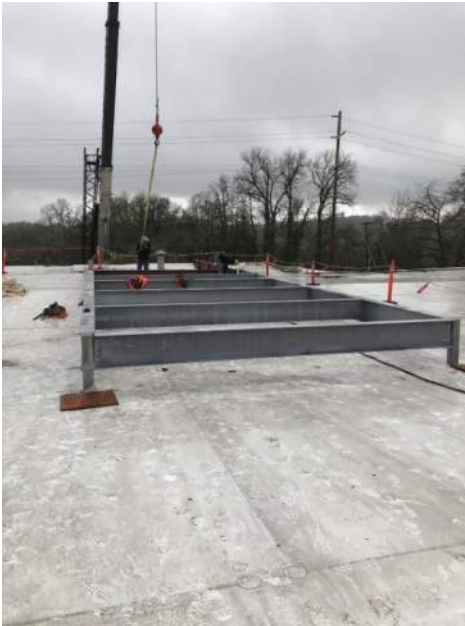
CVHS – HVAC Roof support steel going in through holes in roof deck
