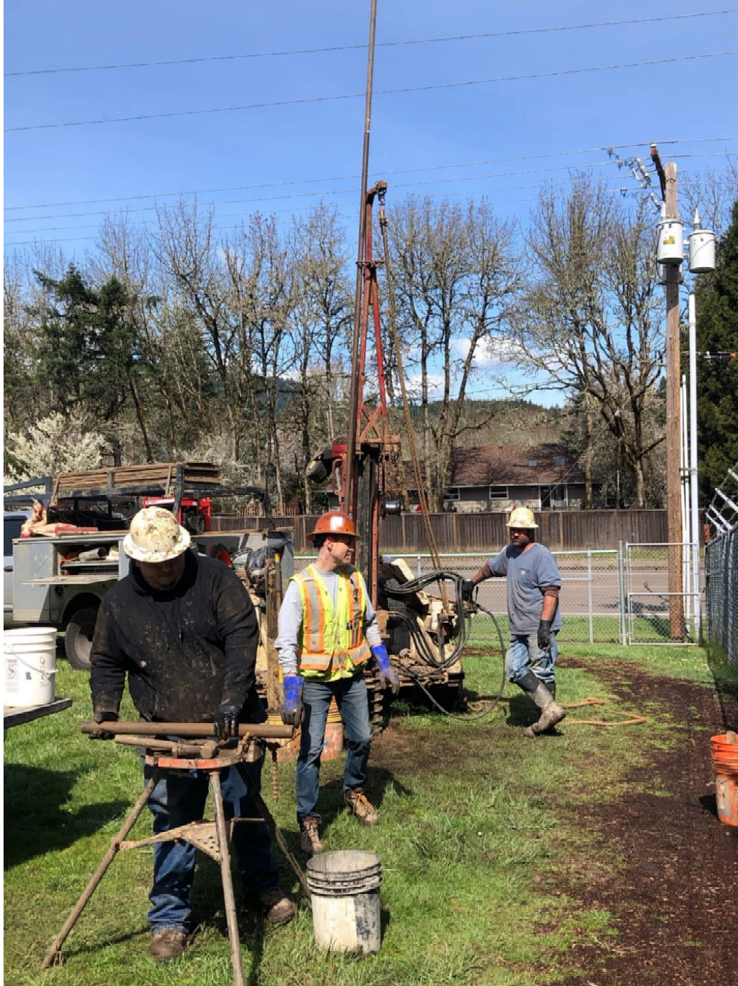
Workers from Foundation Engineering and Western States Drilling performing drilling for geotechnical survey
