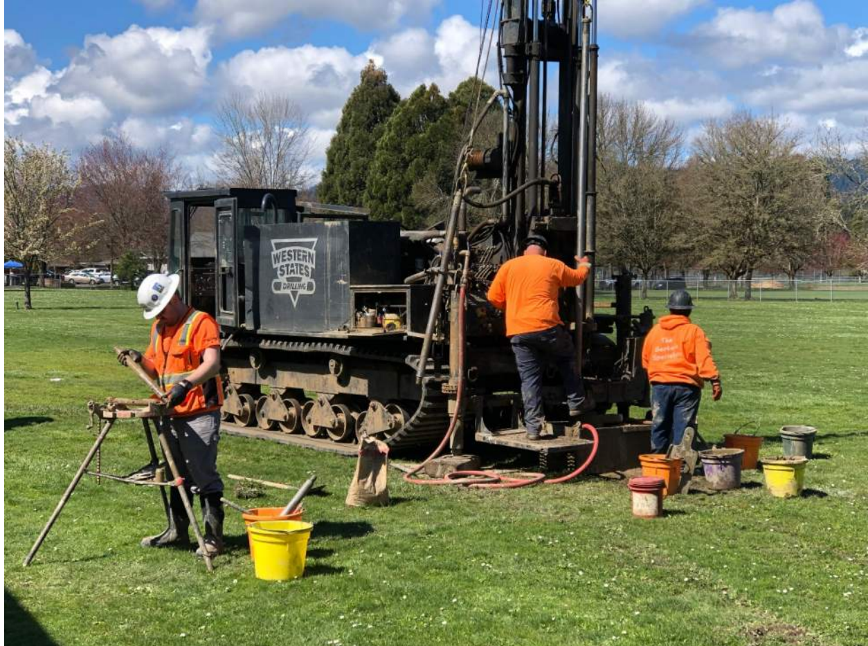
Workers from PBS Engineering and Environmental and Western States Drilling performing the geotechnical survey and associated drilling
