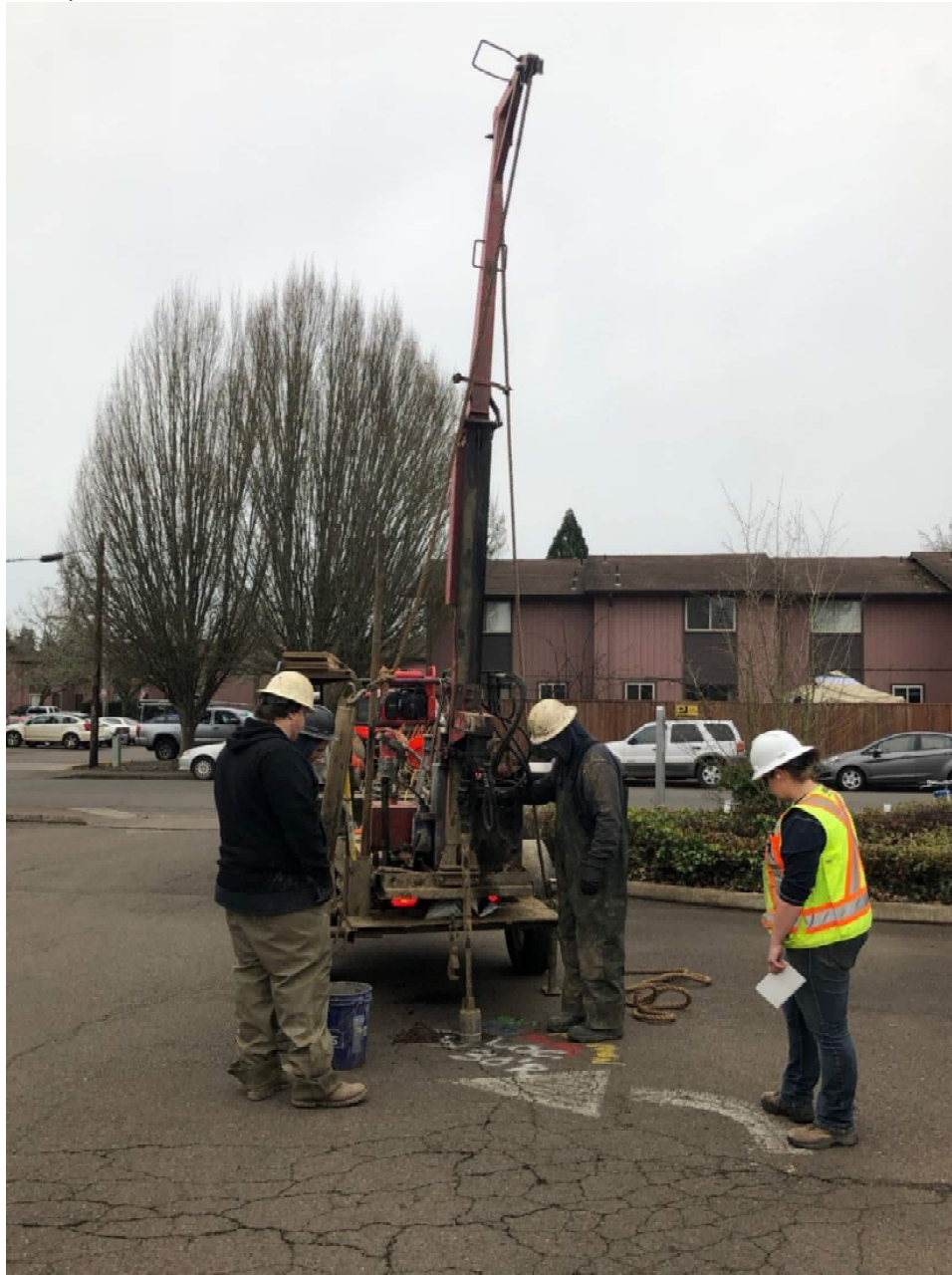
Workers from Foundation Engineering and Western States Drilling perform drilling for the geotechnical survey
