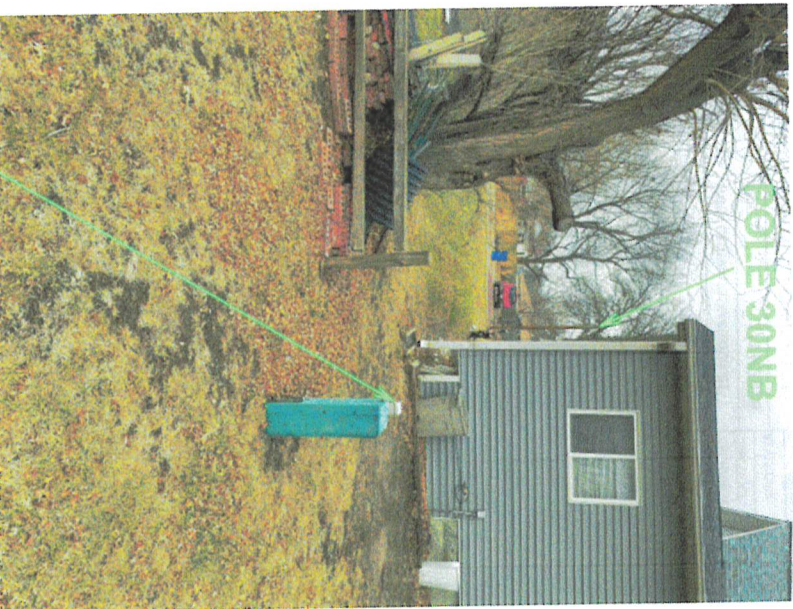
POLE 30NB COPPER PED 35NB LOOKING NORTH
