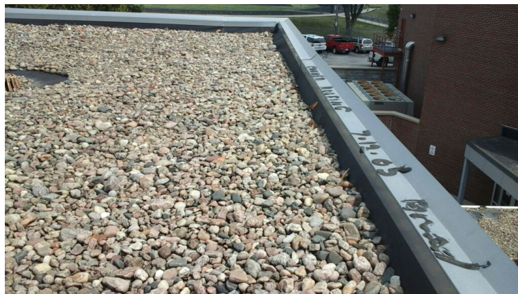
Photo showing condition of perimeter flashings.
