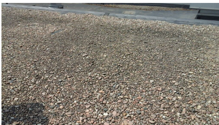
Photo showing evidence of ponding water.
