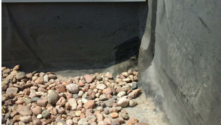
Photo showing tenting occuring in the corner of the perimeter flashings.
