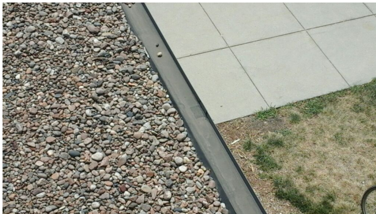
Photo showing condition of the form flashings.
