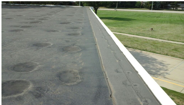
Photo showing condition of the form flashings.
