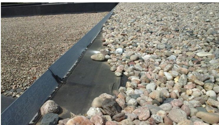
Photo showing condition of the form flashings.
