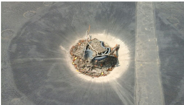
Photo showing clogged drain.
