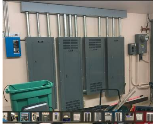
Figure 13 Branch Panels A, B, and C in Electrical Room
