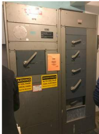
Figure 14 Existing Electrical Service #2
