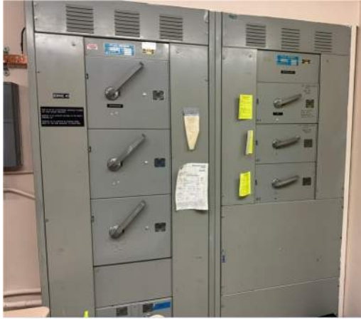
Figure 17 Existing Electrical Service #3
