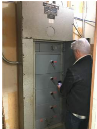
Figure 21 Distribution Panel located in Cafeteria/Gymnasium Area
