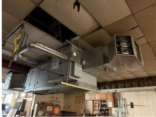
Figure 4 Gas-fired HVUs serve the CTE classroom spaces. These units appear to be in good condition overall and upgrades may not be necessary.
