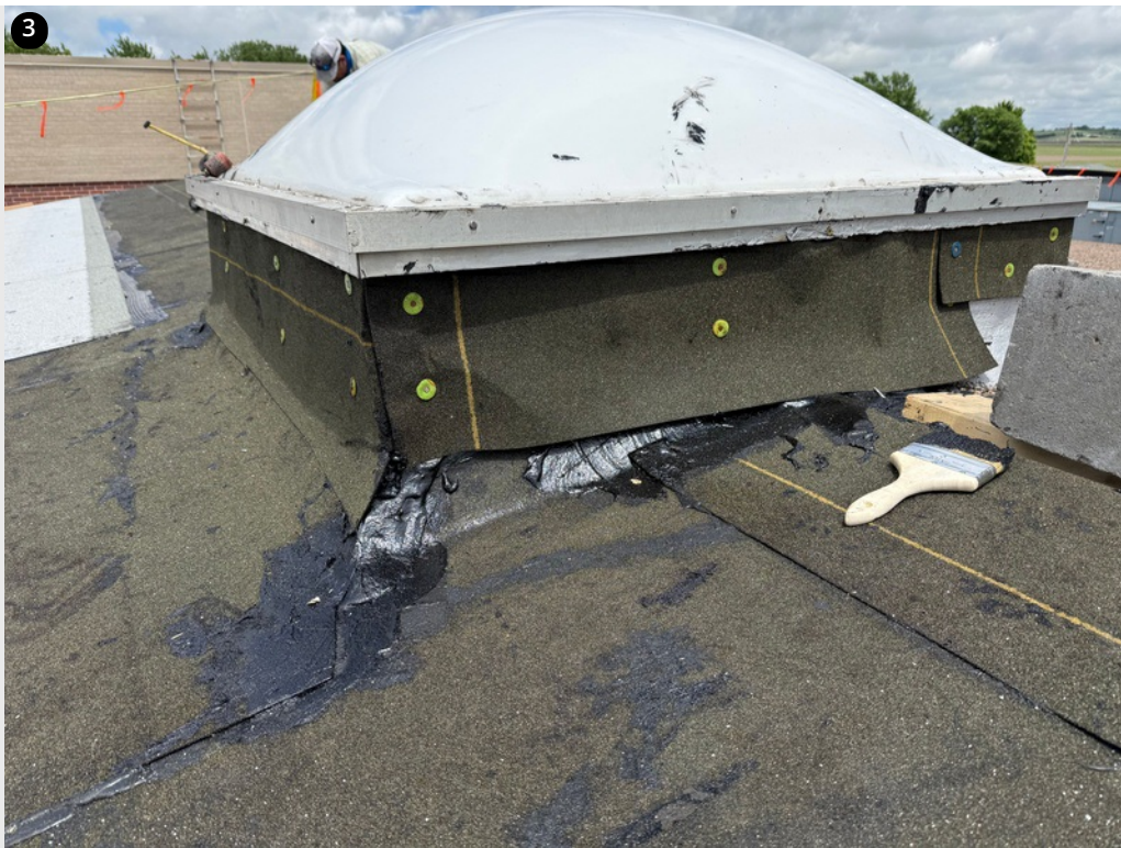
Skylight curb has been raised for proper flashing height.
