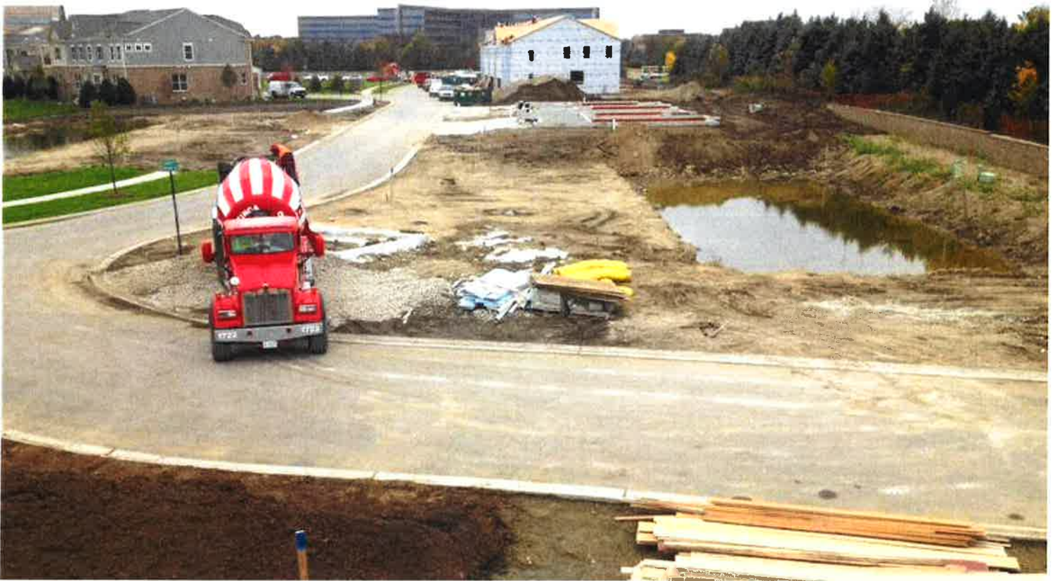
Riverside Road (right) could become the home of new townhomes. Developer Pulte Homes already has started construction near Riverside Road on a different townhome project. (Ronnie Wachter / Pioneer Press)
