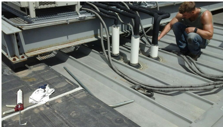
Photo showing multiple projections through roof above major problem area.
