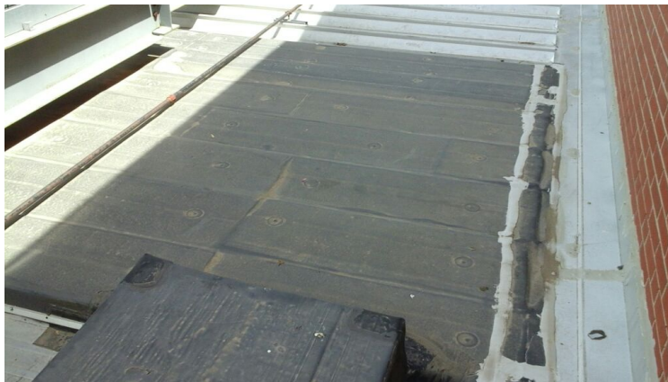
Photo showing additional flute fill in area above HVAC units. The seam should be monitored as it is caulked with same ineffective material through out roof.
