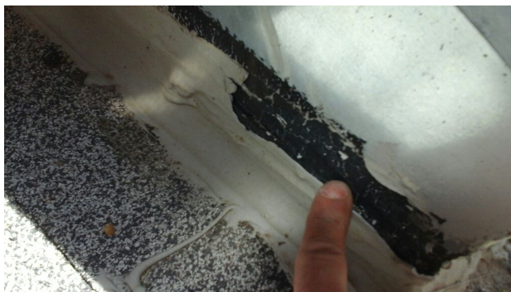
Photo showing another example of caulking not Adhered to metal fully and pulling right up. This is most likely the cause of the leaks below.
