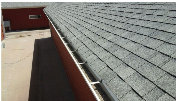
Photo showing condition of the gutter edge.
