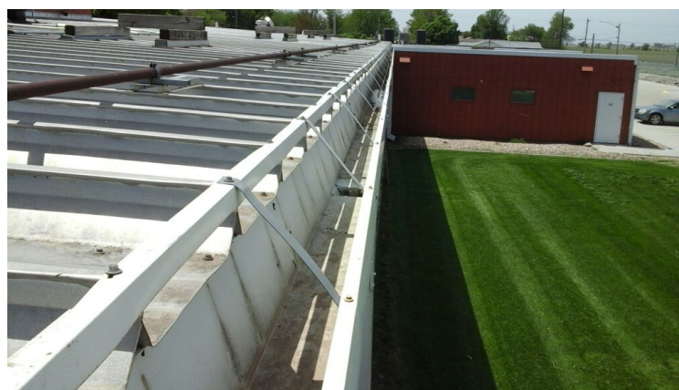
Photo showing condition of the gutter edge. This gutter is appropriately attached with top lower than metal roof.
