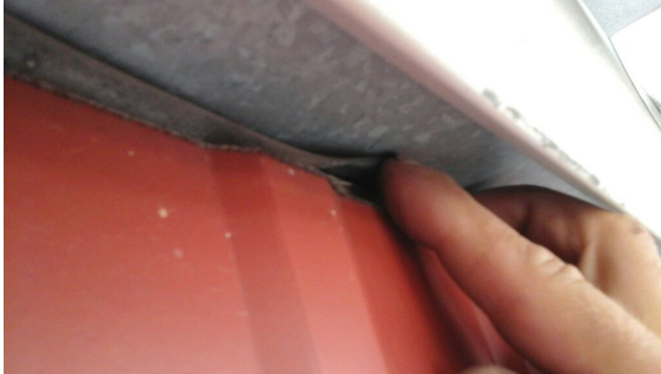
Photo showing area under gutter where rubber does not fully flash wall. Exposed framing underneath.
