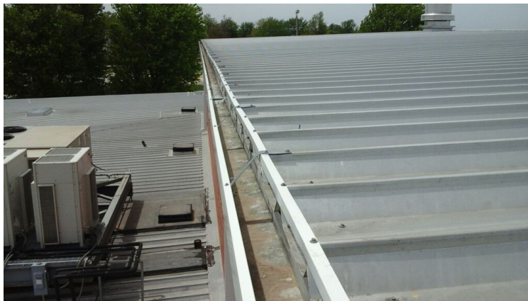
Photo showing condition of the gutter edge.
