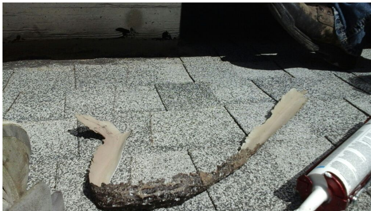
More ineffective caulking that was placed on top of existing caulking. Pulled right up and was doing nothing to prevent water from getting through.
