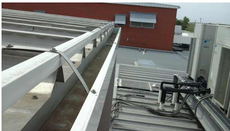
Photo showing condition of the gutter edge. Top of gutter is even with metal roof. Potential back flow issue into area directly below that is exposed.
