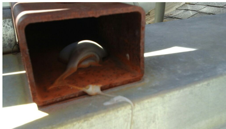
Photo showing bolt into curb covered with caulking.
