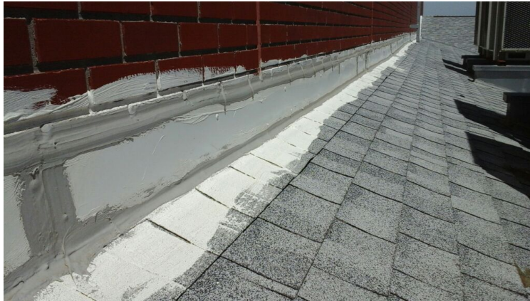
Photo showing condition of the perimeter flashings next to HVAC units. This is an area with heavy leaks reported.
