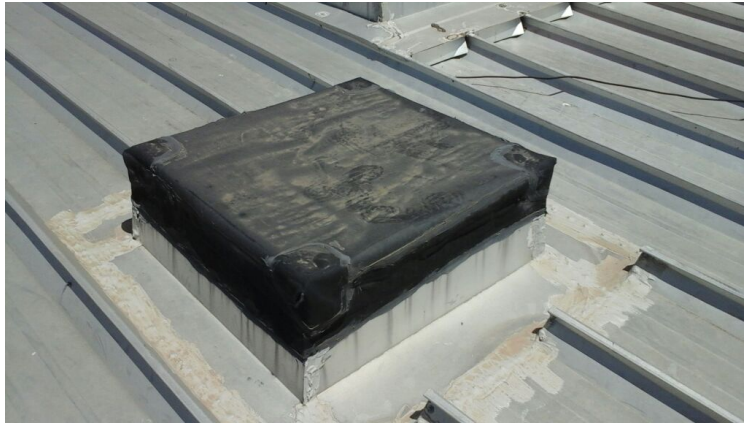
Photo showing condition of unused projection flashings.
