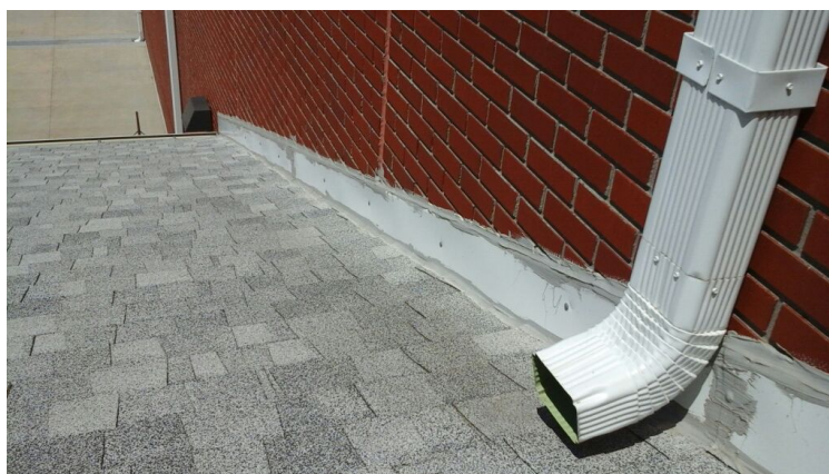
Photo showing condition of the perimeter flashings next to door 02.
