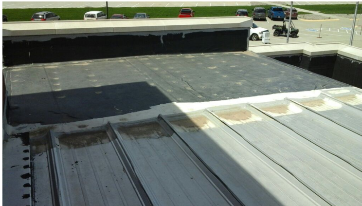
Photo showing joint between rubber and metal roof that is caulked with ineffective long term material.
