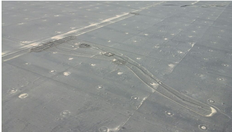
Photo showing wrinkles that were patched in at installation.
