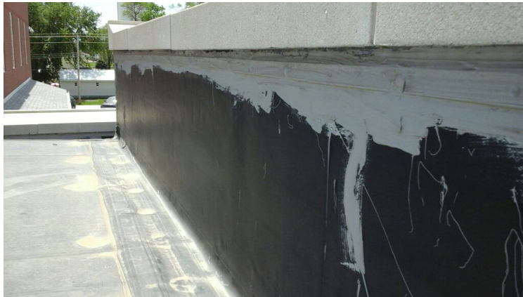
Photo showing ineffective caulking on every joint.
