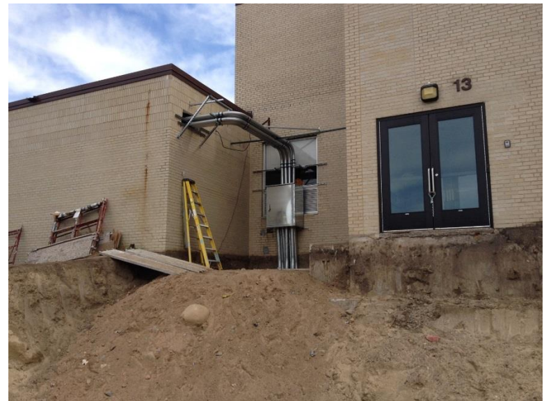
09/05/15 Above grade Conduit routing into the existing facility for the new electrical service.
