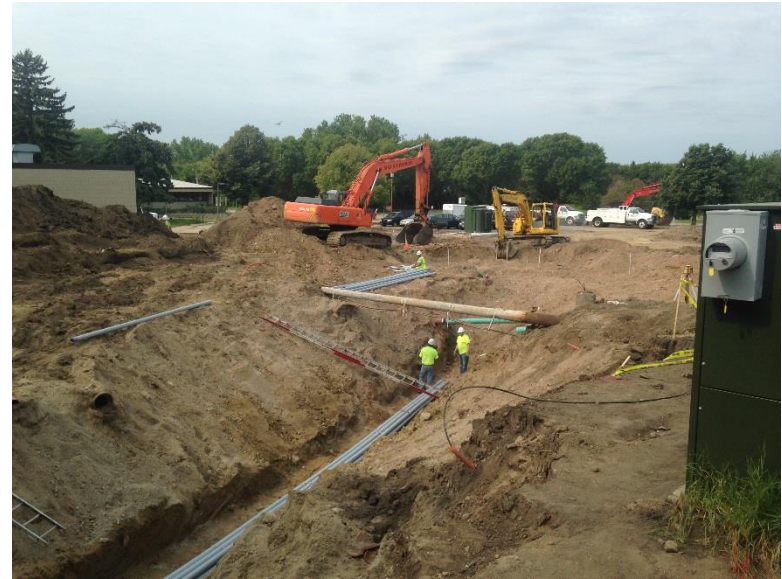
08/27/15 Installing the new underground electrical service below the existing electrical service being supported by the horizontal pole.
