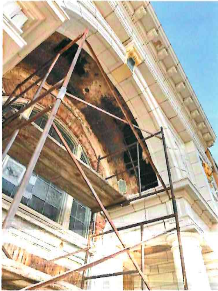
The arched ceiling of the main entrance. At least half of the metal crossbars of the skeleton had rusted so badly, they were no longer embedded in the brick and therefore provided no structural support.
