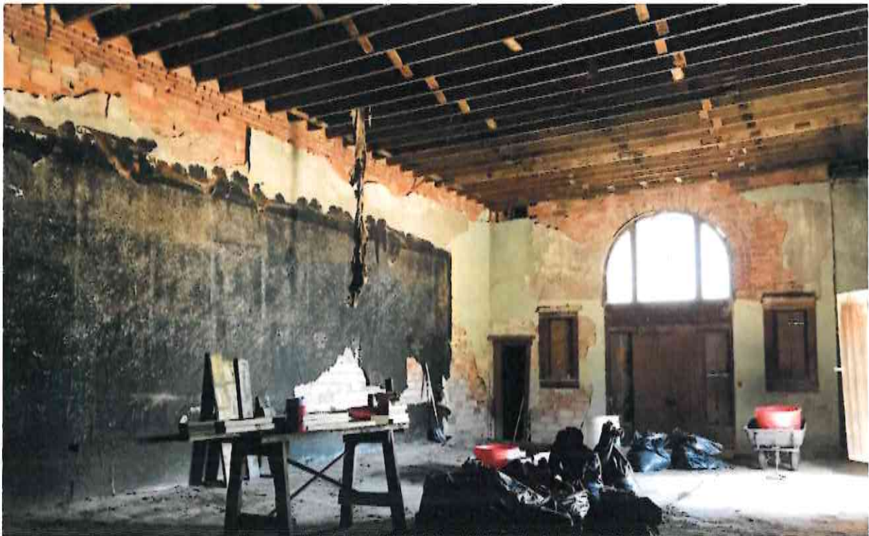
The main room of the interior, looking southeast. All the plaster was crumbling or covered in black tar paper, the wood trim was mostly rotten, and the floor had 18" of concrete and filler poured over it.
