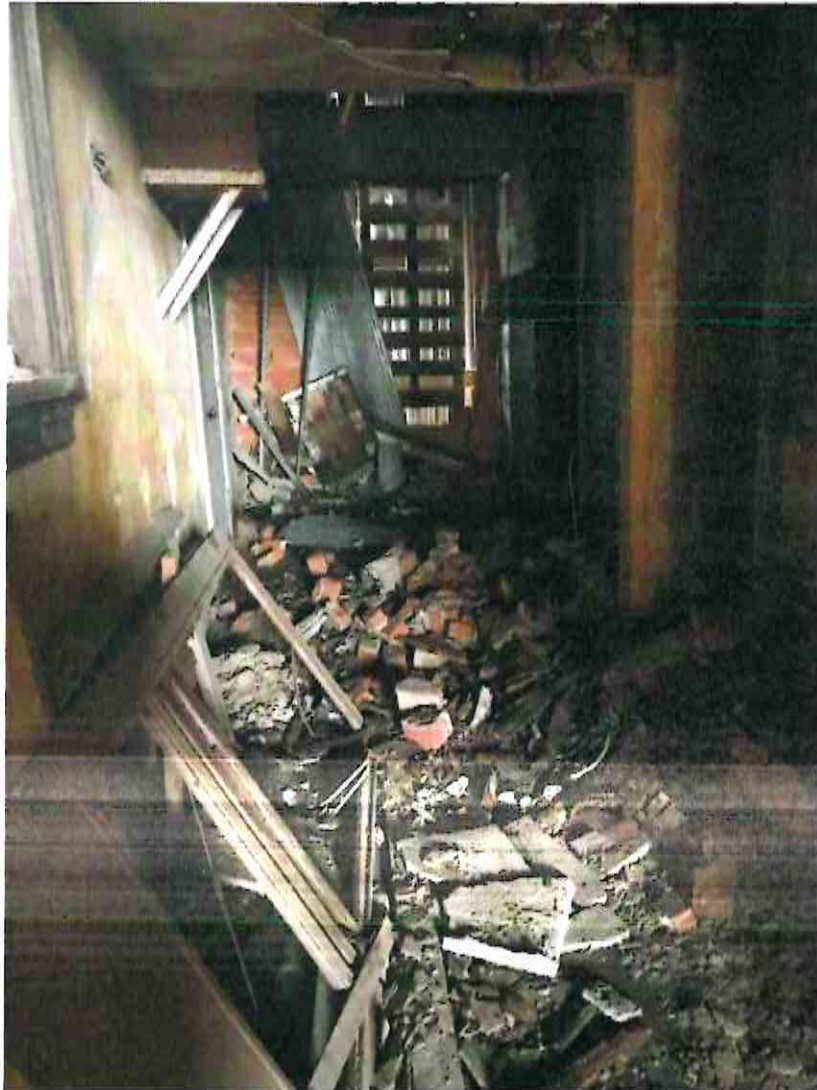
Debris that had piled up over the years in the hallway to the rear door of the building.
