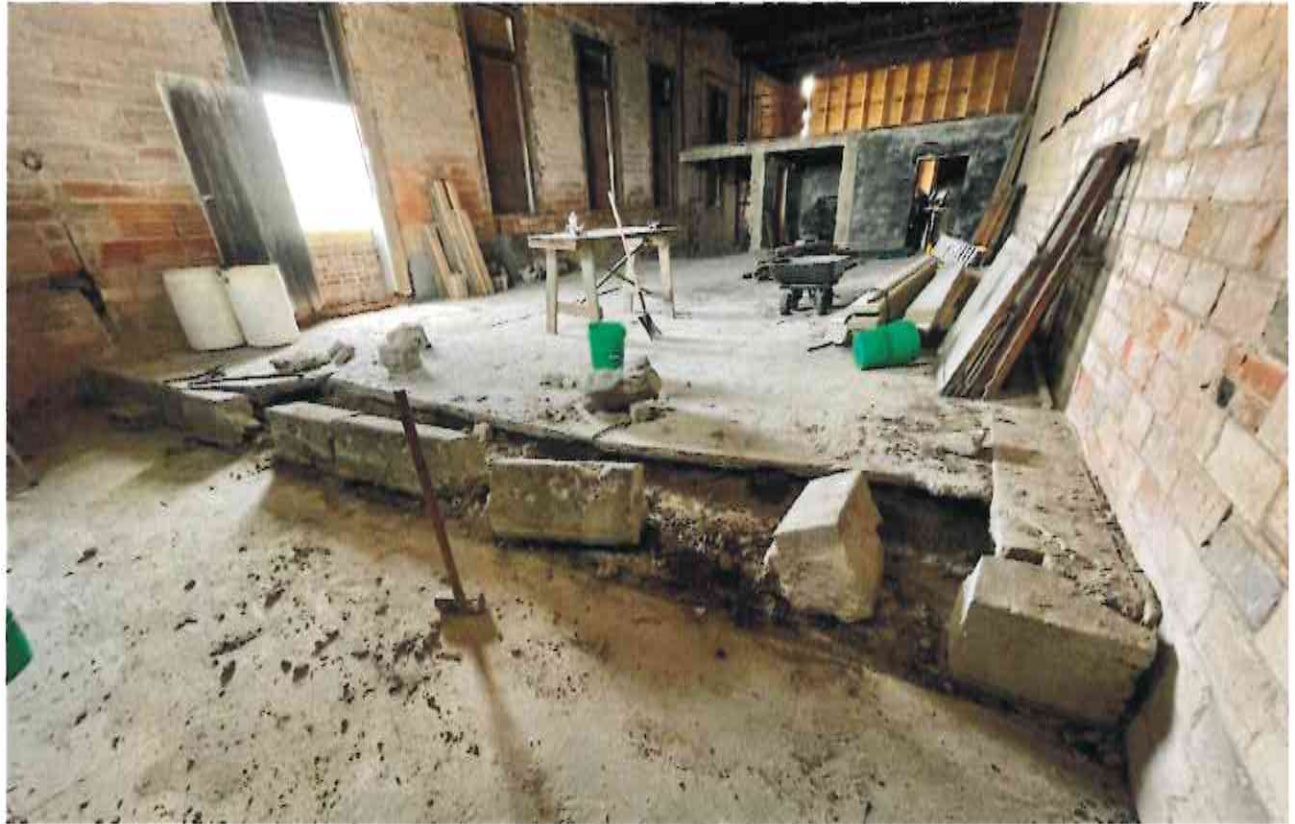
Starting removal of the cement and filler that had been added over the original floor.
