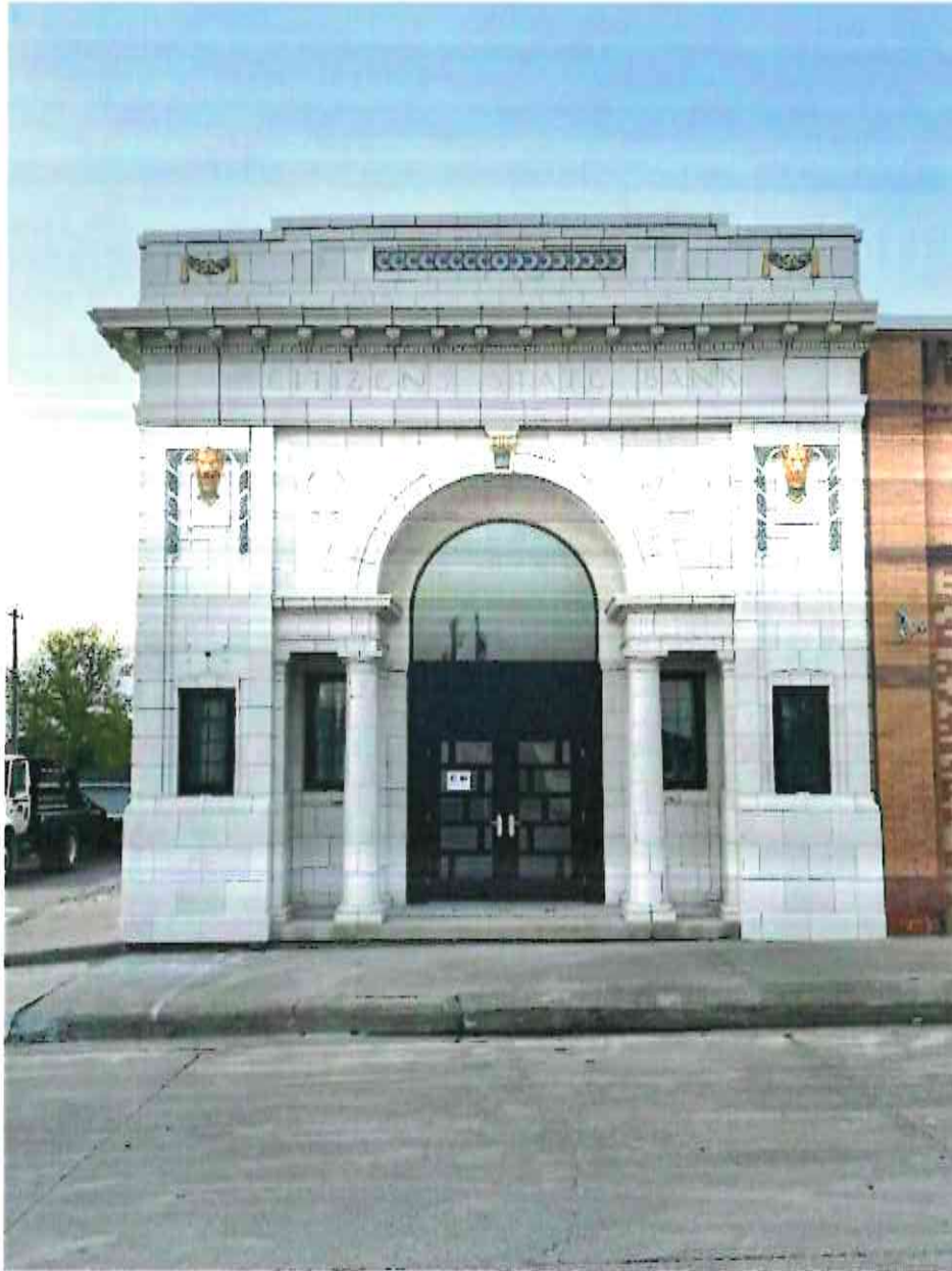
The front/south of the building, with all new windows and doors, and stucco for the arched entrance and alcove ceilings.
