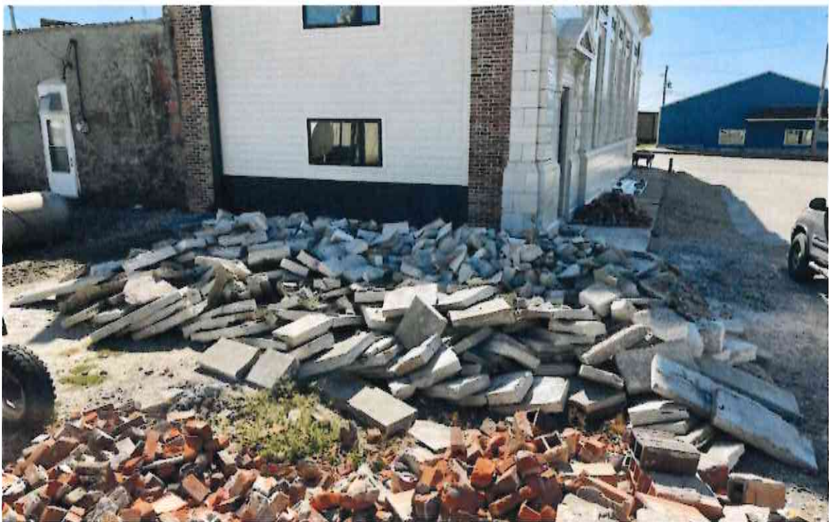
All the concrete that had been removed from the main room pictured above.
