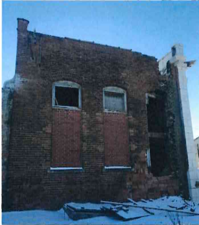
The rear/north wall. The drainage from the roof was funneled to the top right corner, and with no downspout, water just ran down the wall for years.
