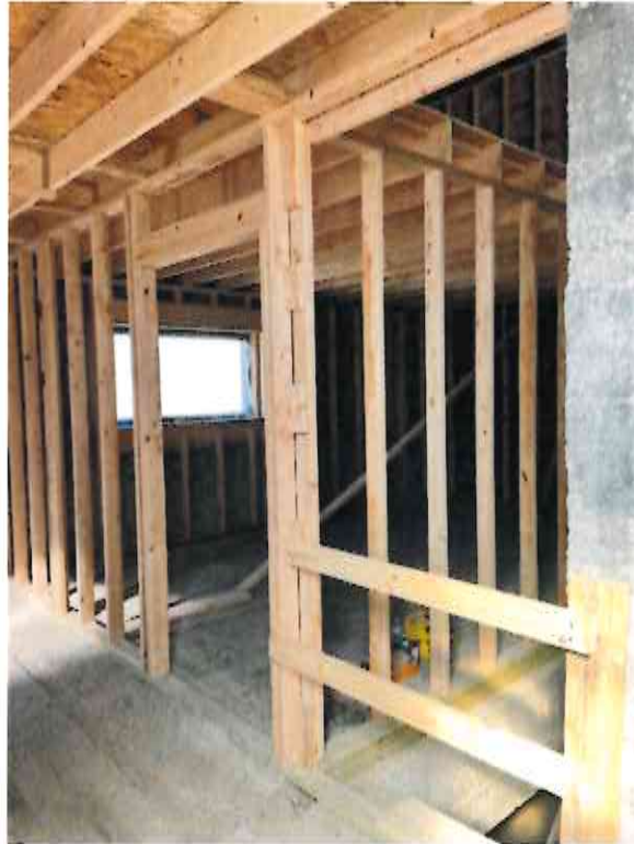
At the north end of the building, this framing was added in anticipation of this space becoming the kitchen or restrooms for the main event space.
