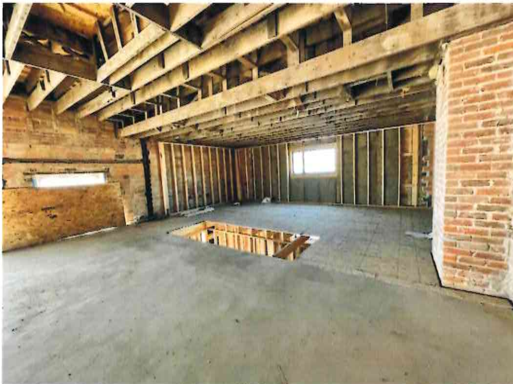
Standing at the southeast corner of the mezzanine, looking northwest. The foreground (cement floor) is original, while the particle board is extending the mezzanine over the added rooms below.
