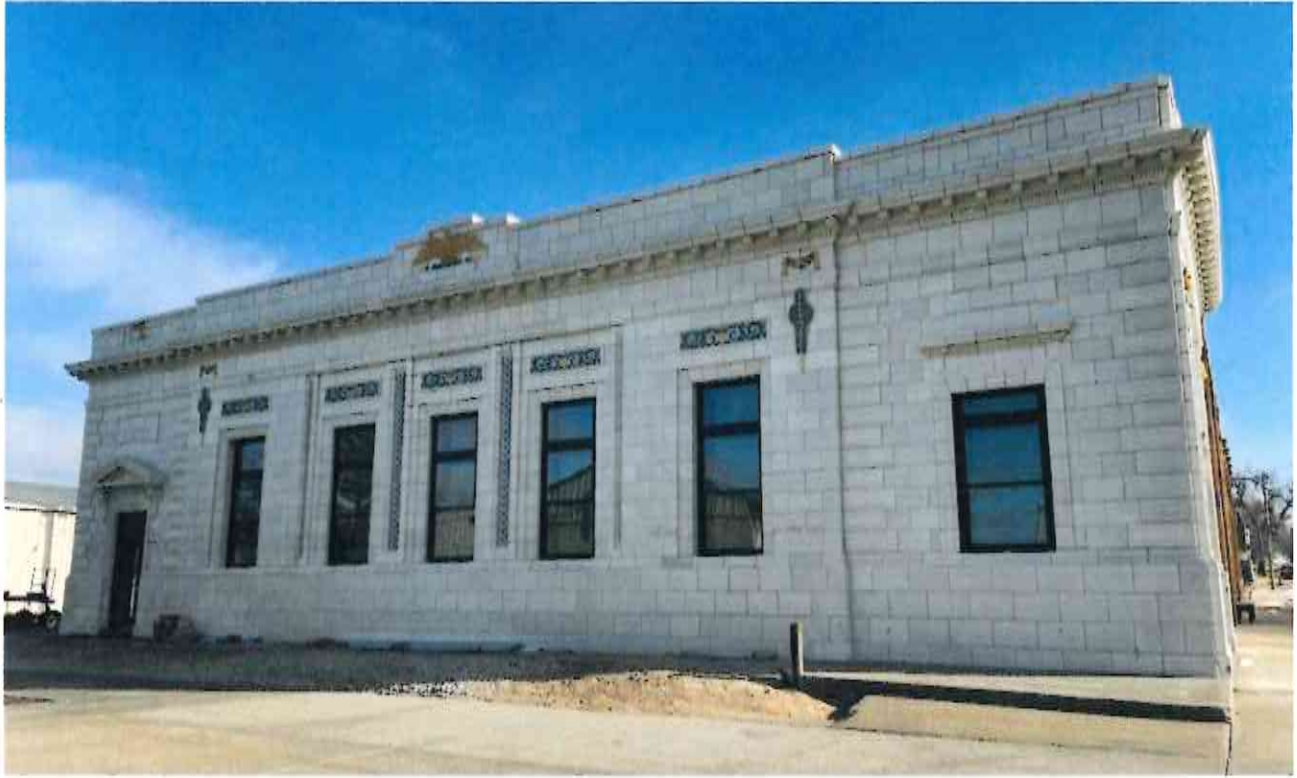
The west side of the building. The one window (second from right) was restored back to a window, then all new windows and one new door were installed.
