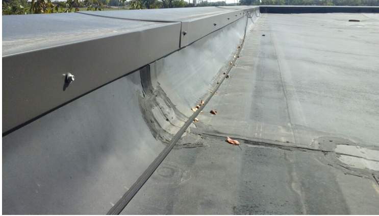
Photo showing tenting occurring along the perimeter flashings.
