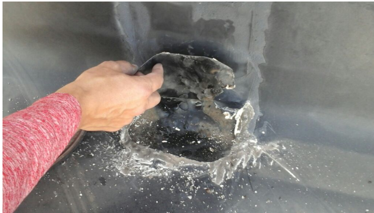
Photo showing a patch in the perimeter flashing where was glued down with caulking. Pulled up as part of the maintenance agreement.
