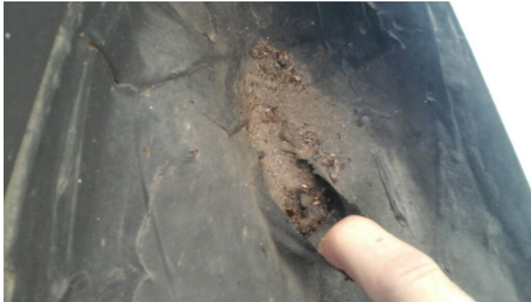
Photo showing a hole in the projection flashing blowout patch. Repaired as part of the maintenance agreement.
