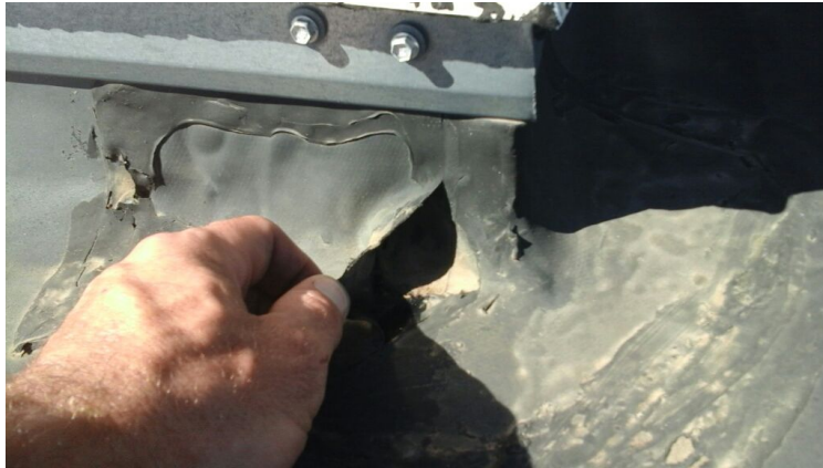
Photo showing patch pulling loose on the hatch flashing. Repaired as part of the maintenance agreement.
