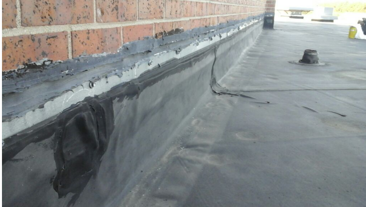
Photo showing poorly terminated perimeter flashings. The insulation all along this wall is soft.
