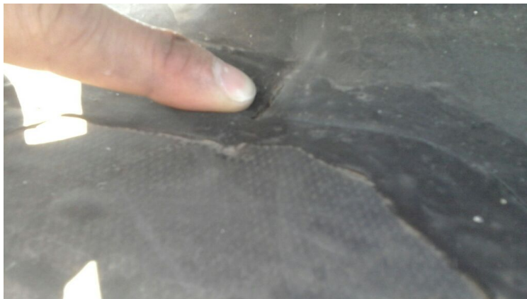
Photo showing a hole in the projection flashing. Repaired as part of the maintenance agreement.
