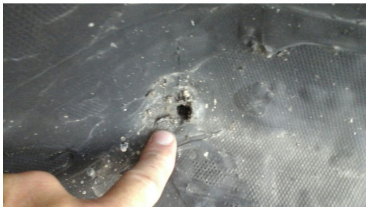
Photo showing a hole in the perimeter flashing. Repaired as part of the maintenance agreement.
