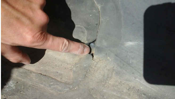
Photo showing a hole in the perimeter flashing. Repaired as part of the maintenance agreement.
