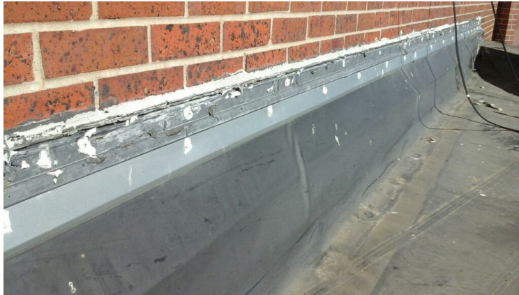
Photo showing perimeter flashing with no termination. The only thing preventing water from entering the building is the caulking which is beginning to fail. The old caulking was removed and replaced as part of the maintenance agreement.
