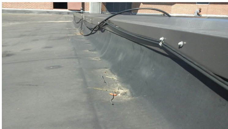
Photo showing tenting along the perimeter flashings.
