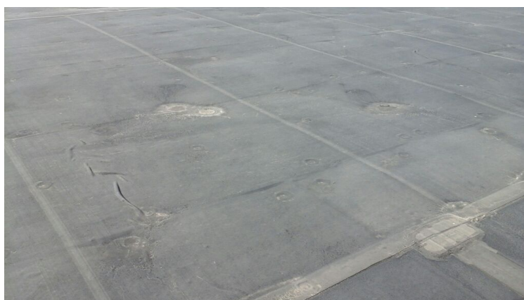
Photo showing wrinkles in the field membrane.
