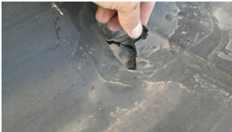
Photo showing blowout patch on a seam pulling loose. Repaired as part of the maintenance agreement.
