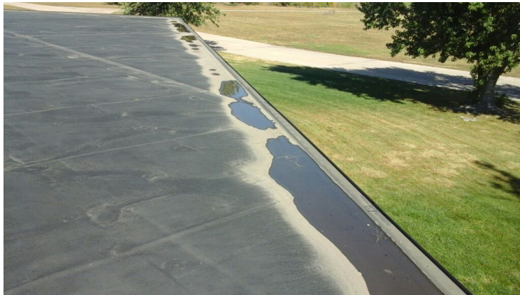
Photo showing additional ponding water along the perimeter edge.
