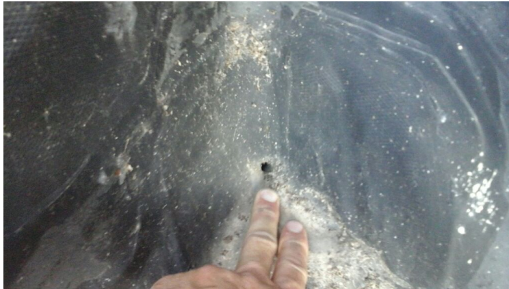
Photo showing a hole in the perimeter flashing.
