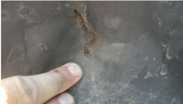
Photo showing a hole in the perimeter flashing. Repaired as part of the maintenance agreement.
