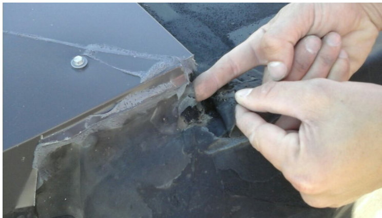
Photo showing a hole in the expansion joint. Repaired as part of the maintenance agreement.
