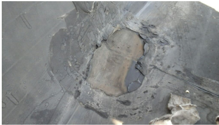
Photo showing a blowout patch that pulled up. Repaired as part of the maintenance agreement.
