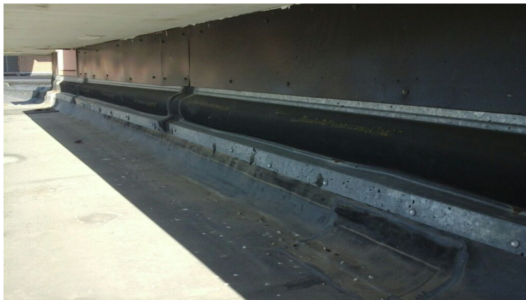
Photo showing condition of expando flash joint along penthouse perimeter.
