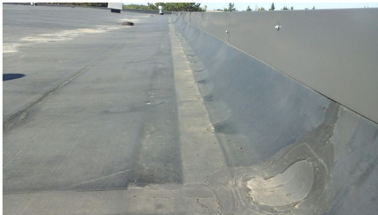
Photo showing tenting along the perimeter flashings.
