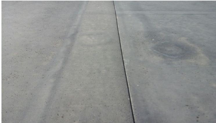
Photo showing seam lacking proper seam tape overlap. This seam is also a backward lap so that the seam is open to the peak.
