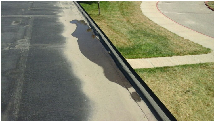
Photo showing ponding water along the perimeter edge.
