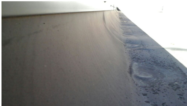
Photo showing tenting along the perimeter flashings.
