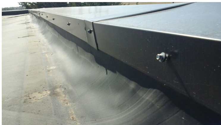
Photo showing metal fasteners backing out.
