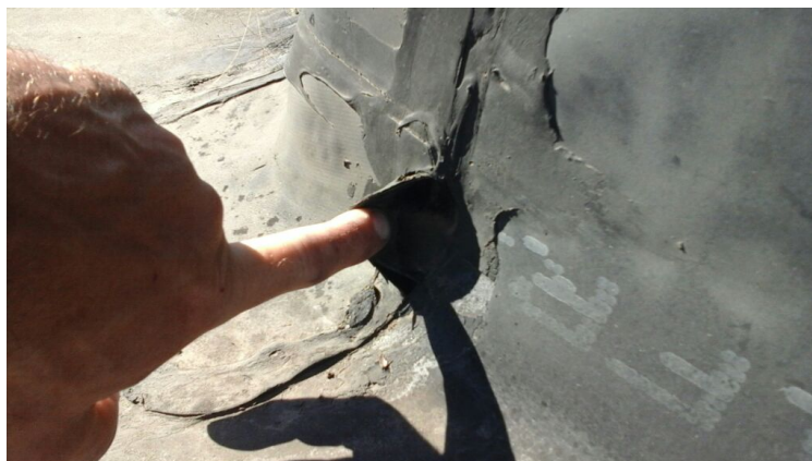
Photo showing a hole in the field membrane. Repaired as part of the maintenance agreement.
