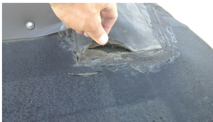
Photo showing form flashings beginning to pull loose. Repaired as part of the maintenance agreement.
