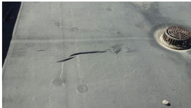
Photo showing a wrinkle in the field membrane.
