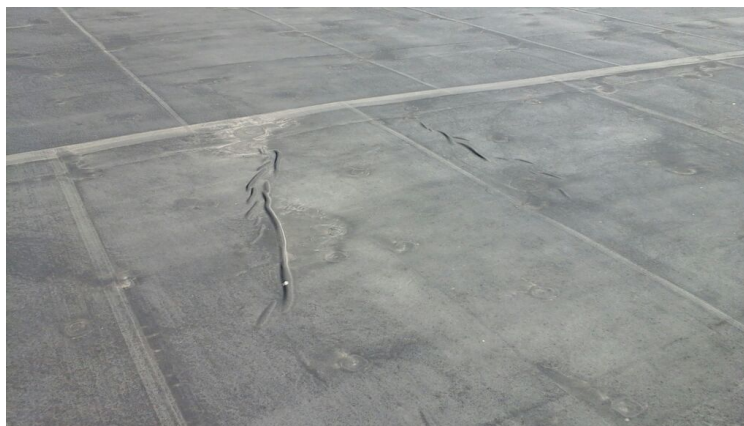
Photo showing wrinkles in the field membrane.
