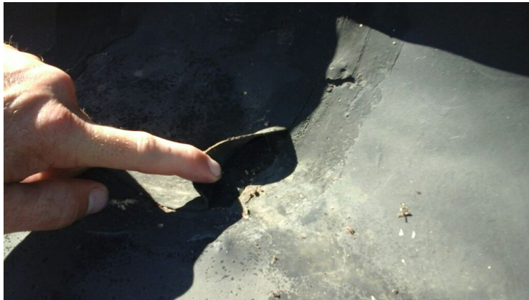
Photo showing hole in the perimeter flashings. Repaired as part of the maintenance agreement.
