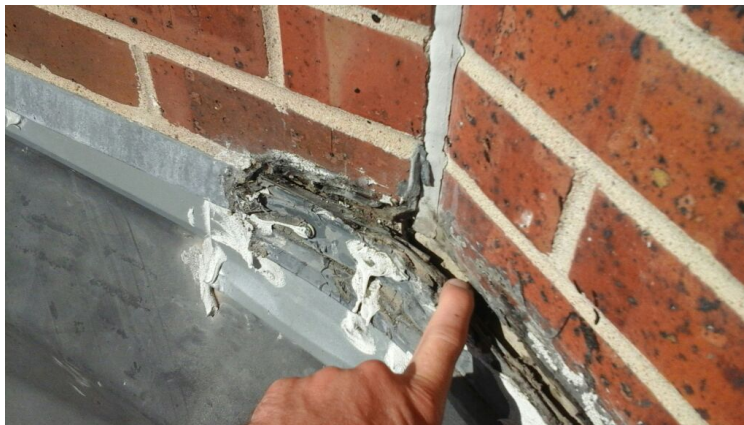
Photo showing a gap in the perimeter flashing that is causing a leak. Repaired as part of the maintenance agreement.
