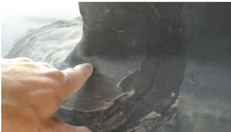
Photo showing a hole in the projection flashing. Repaired as part of the maintenance agreement.
