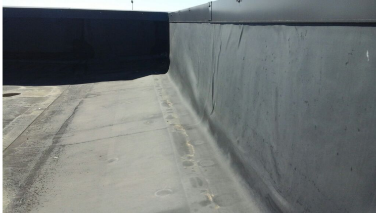
Photo showing perimeter flashings beginning to delaminate.
