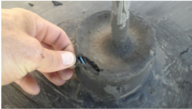
Photo showing a pitch pan that is deteriorating. Repaired as part of the maintenance agreement.
