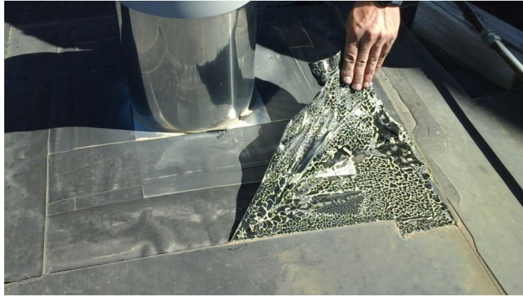
Photo showing tape used as flashing pulling up. Repaired as part of the maintenance agreement.
