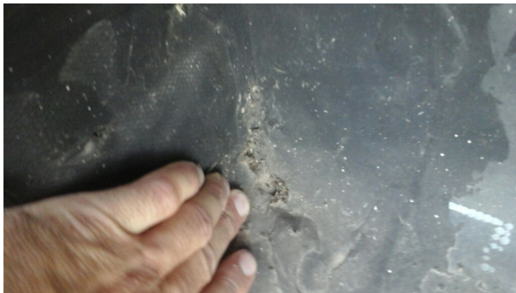
Photo showing a hole in the perimeter flashing. Repaired as part of the maintenance agreement.
