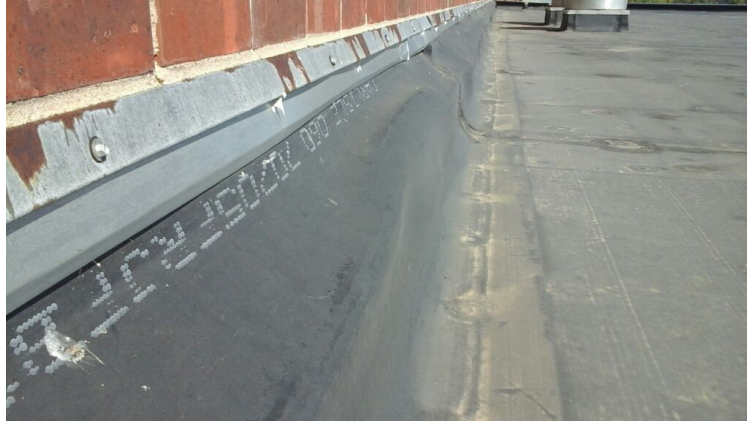
Photo showing condition of perimeter flashing that was installed over the top of another perimeter flashing.
