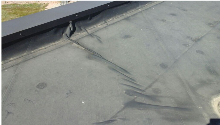
Photo showing wrinkles in the perimeter flashings.
