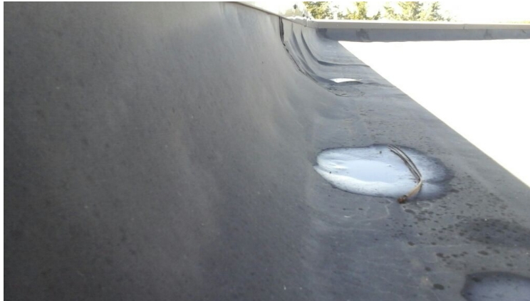
Photo showing tenting along the perimeter flashings.
