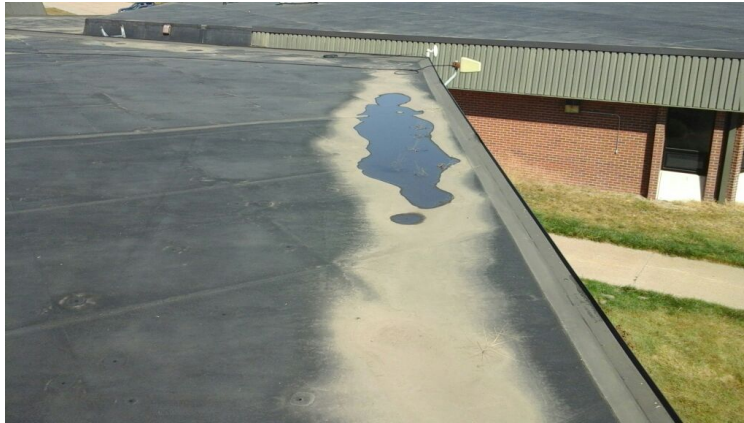
Photo showing ponding water along the perimeter.
