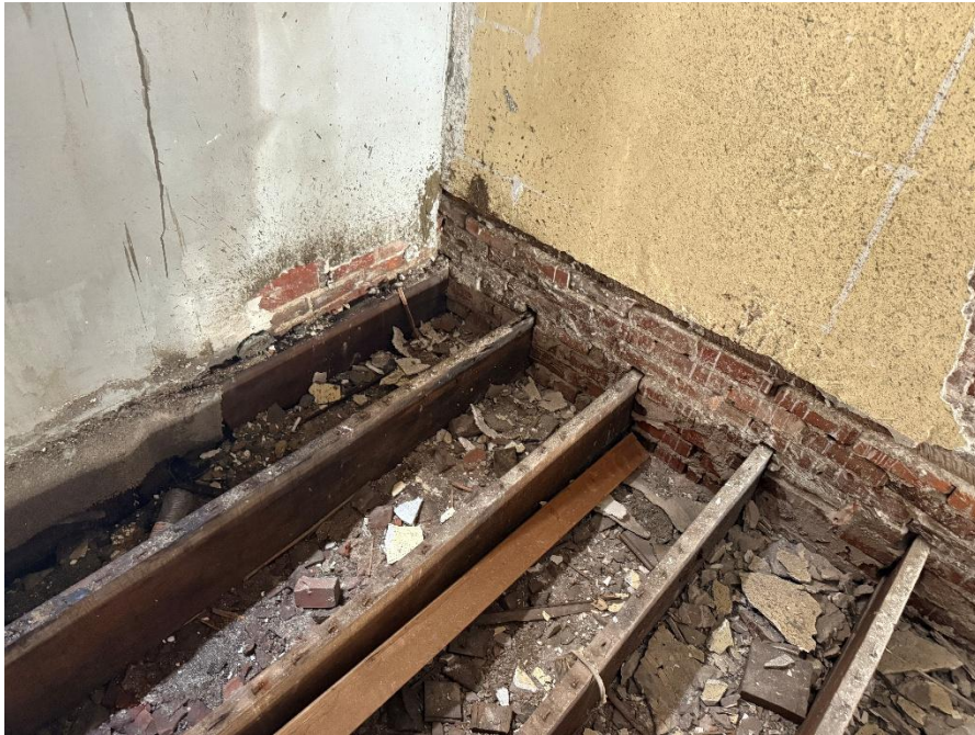
Photo 15 - Second first floor joists in from the west wall at the north building.
