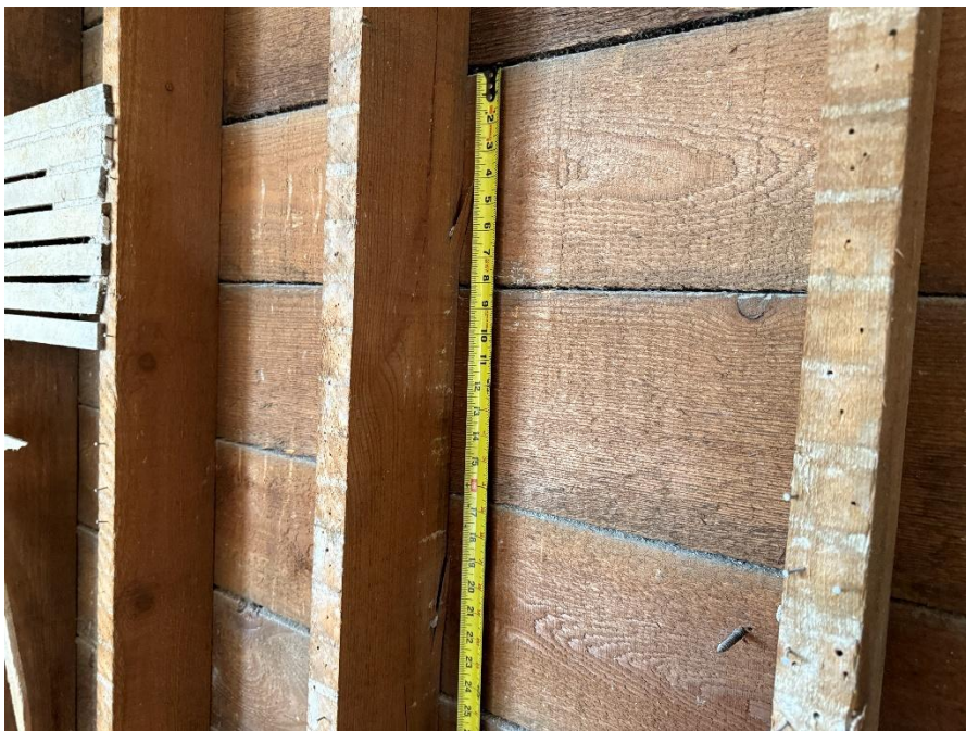
Photo 8 - Lag screws exposed at south wall.
