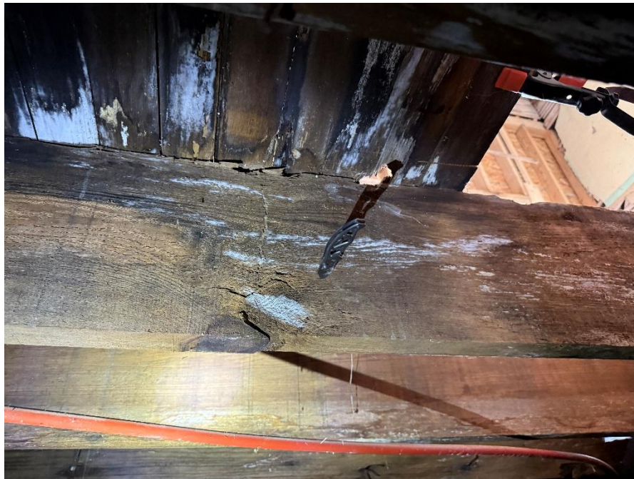
Photo 14 - Split first floor joist.
