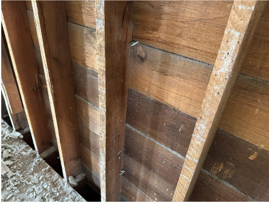
Photo 9 - Exposed lag screws at south wall.
