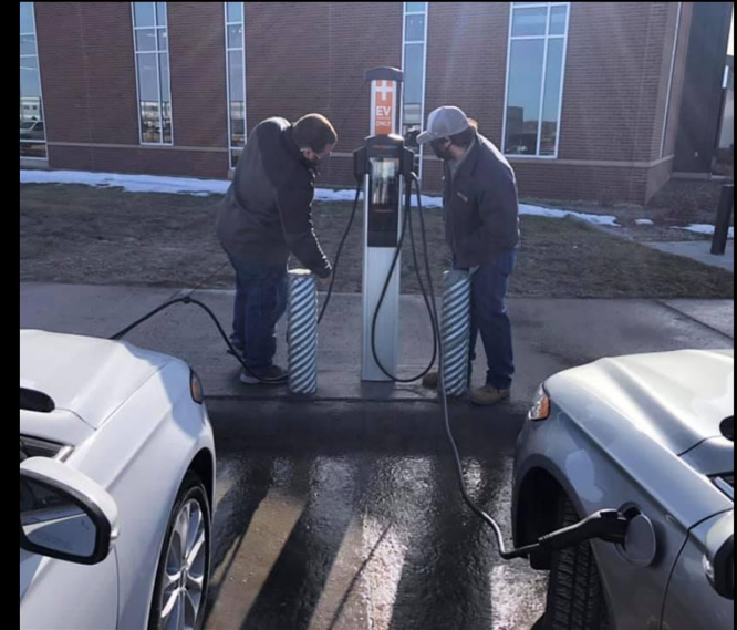
CCC Kearney Center Charging Station
