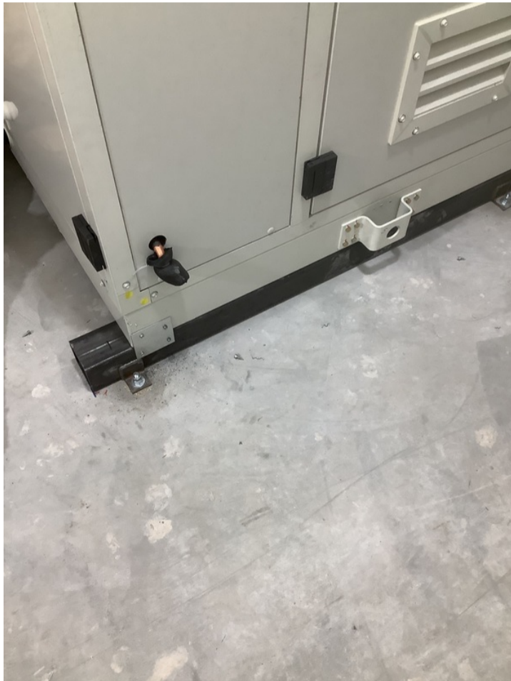
2020-05-28 08:28:08 Vibration isolation on AHU
