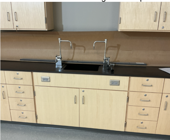
Casework and Plumbing in the Science Room
