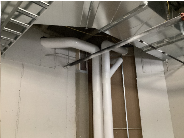
HVAC Plumbing and Electrical
