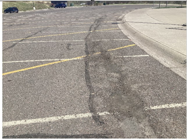
Needed pavement repairs
