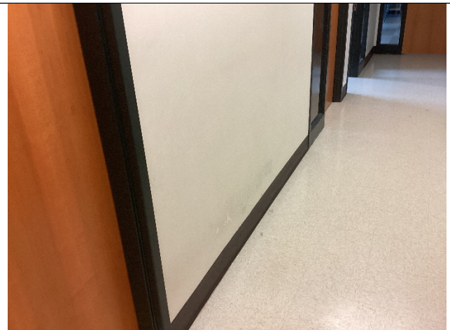
Scuffs on painted surfaces
