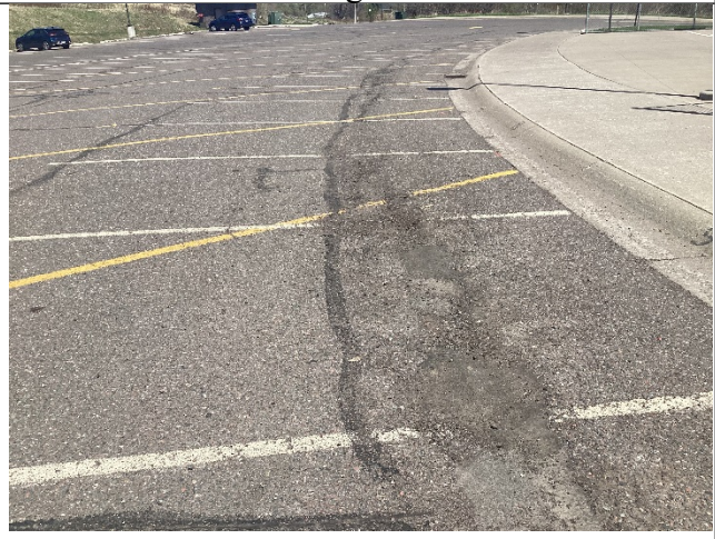
Needed pavement repairs
