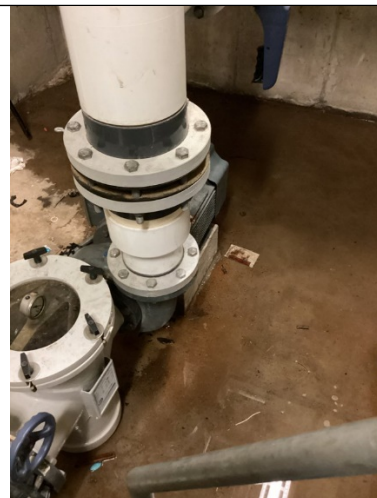
Leaking main pool pump
