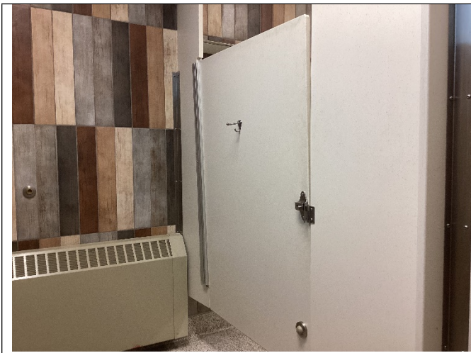
Damaged restroom partition
