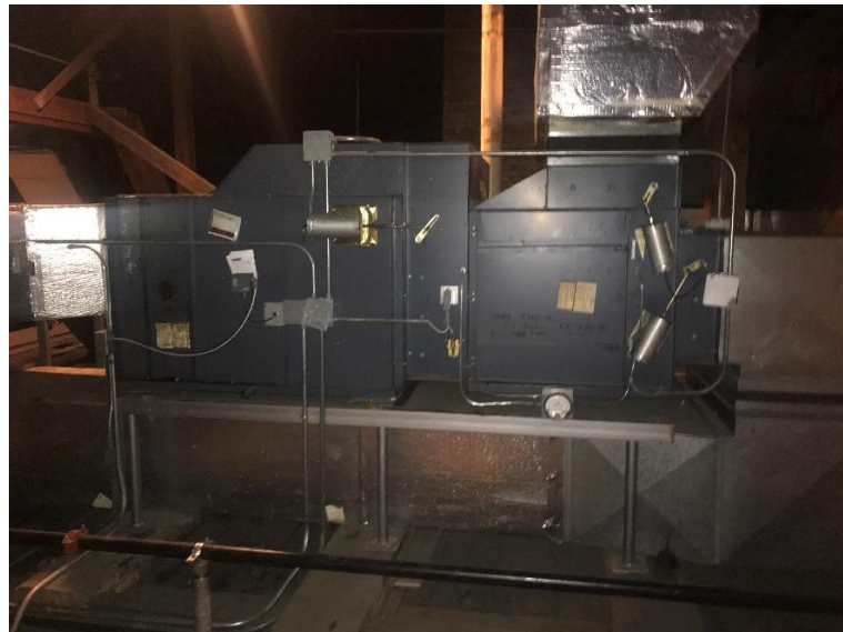
PNEUMATIC DAMPER ACTUATION
