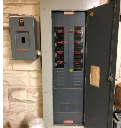
Photo 2: Obsolete Electrical Panel
