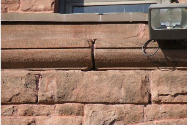
Photo 7: Poor condition mortar joints
