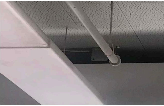
Photo 3 – Upright Sprinkler Heads
