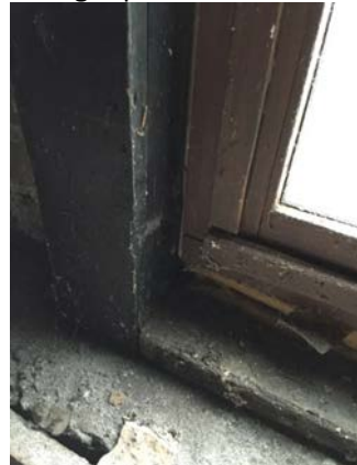
Photo 4: Failed single-pane attic windows
