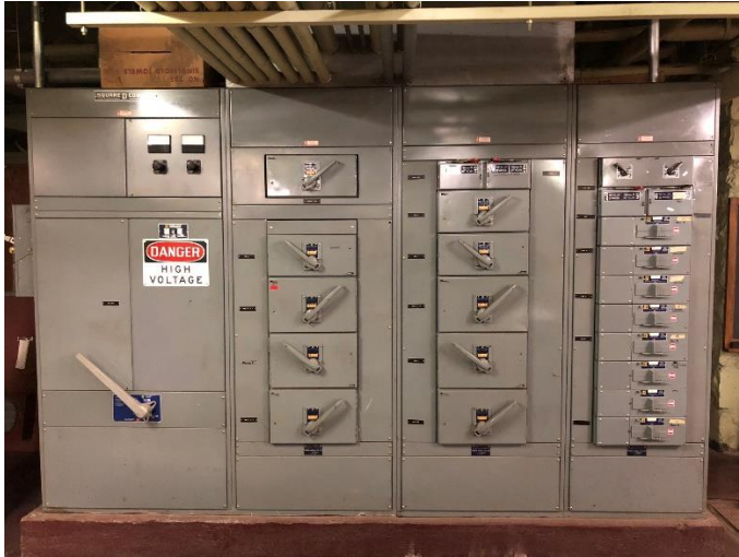
EXISTING 120/208V 3000A FUSED SWITCHGEAR
