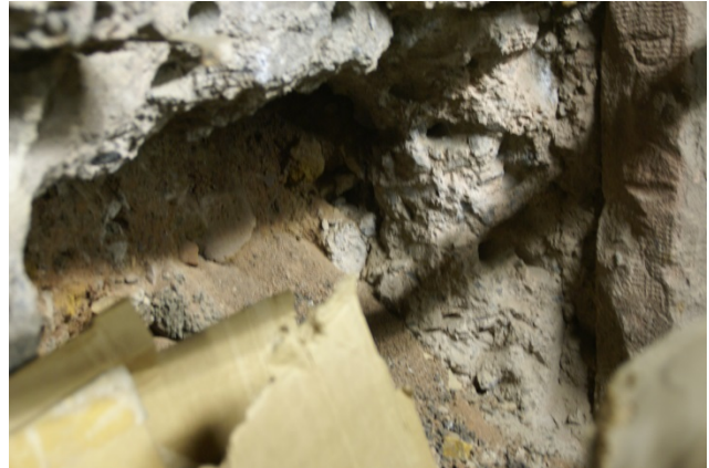
Photo 6: Loading Dock washout
