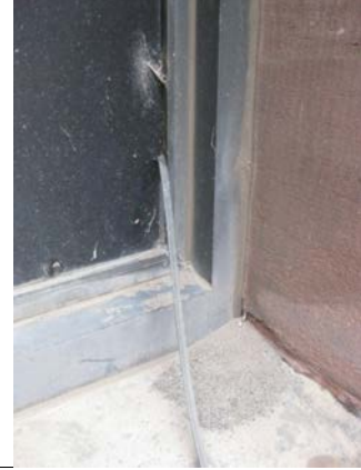
Photo 2: Failed glazing gaskets
