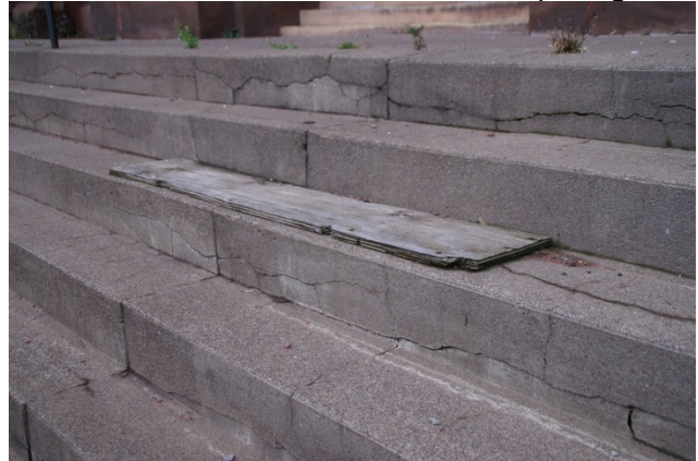
Photo 6: Cracked concrete and covered opening
