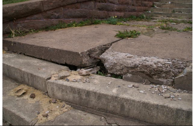
Photo 8: Displaced, cracked, and deteriorated stairs
