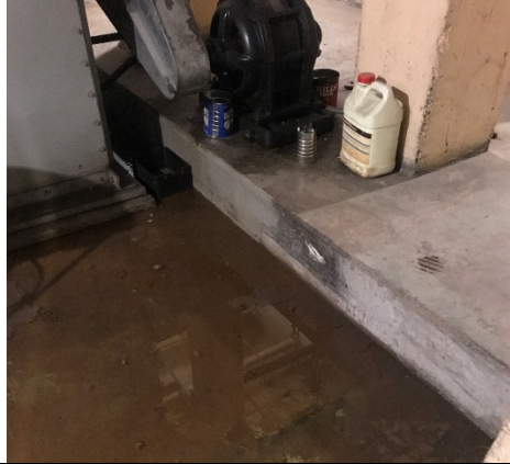
Photo 2 Ground Water in Mechanical Rooms
