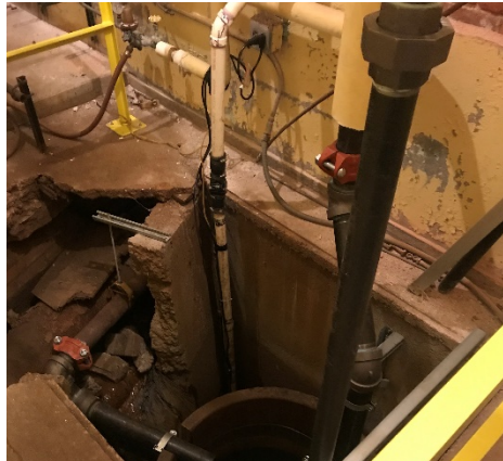
Photo 4 Ground Water & Steam Condensate
