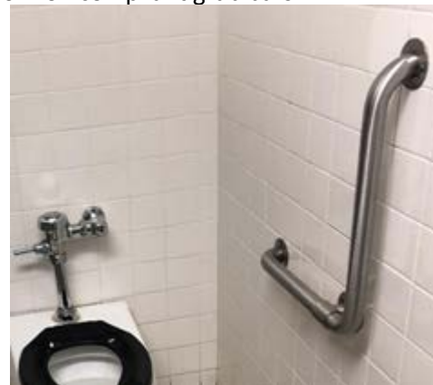
Photo 6 Non compliant grab bars
