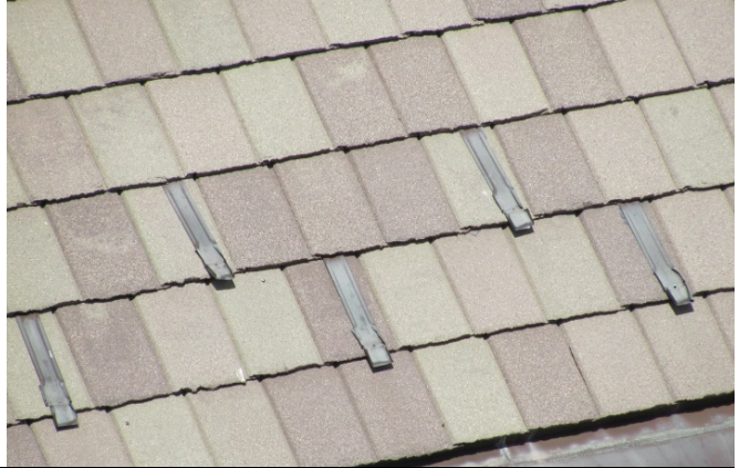
Photo 2: Damaged snow retention system
