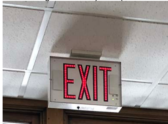
Photo 6: Exit Sign with battery backup
