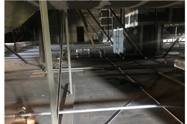
Photo 5 – Attic Dry Pipe System
