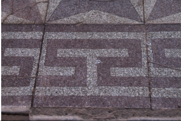
Photo 1: Cracked terrazzo tiles
