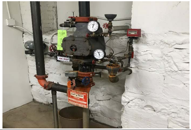
Photo 2 – Dry Pipe Valve
