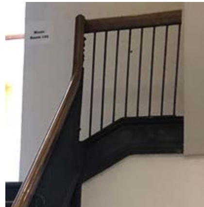
Photo 4 Stair Guardrails – Too low
