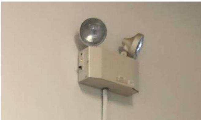
Photo 5: Egress Lighting with battery backup
