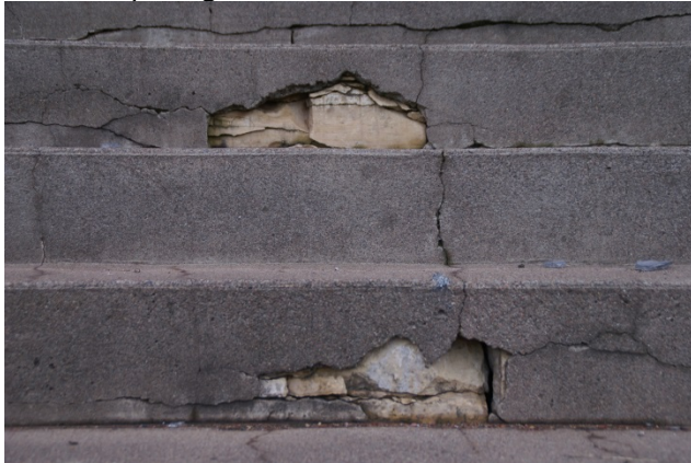
Photo 5: Spalling concrete over limestone stairs
