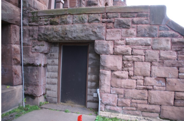
Photo 7: Deteriorated mortar and stone in side wall
