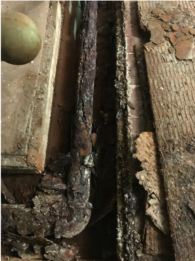
FAILED CONDENSATE LINE
