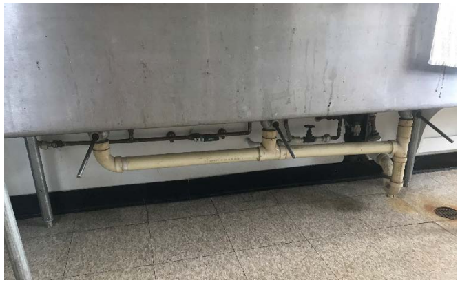
Photo 4 No Grease Trap, PVC
