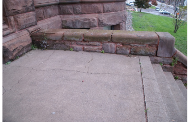
Photo 8: Deteriorated mortar and stone in side wall
