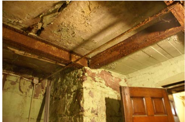
Photo 4: Corroded steel and efflorescence build-up
