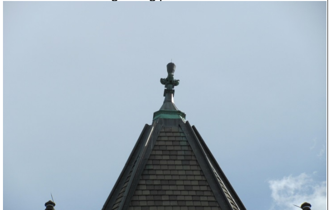
Photo 4: Current lightning protection
