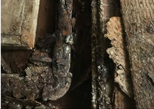
Photo 1 Failed Steam Condensate Pipe
