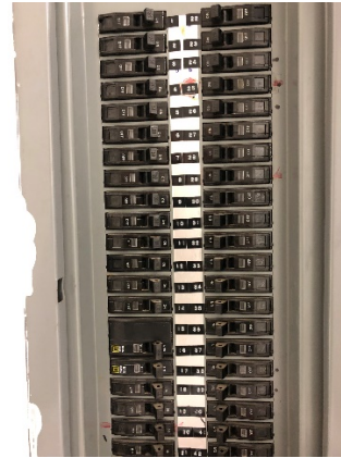
Photo 6: Full Electrical Panel
