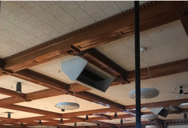
Photo 6 – Board Room Sprinklers
