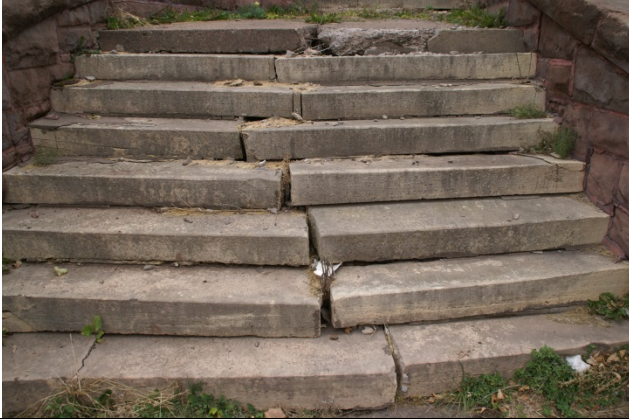
Photo 7: Displaced, cracked, and deteriorated stairs
