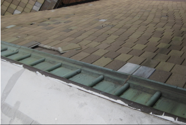
Photo 1: Missing roof tiles
