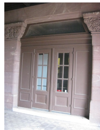
Photo 6: Poor condition side doors at main entrance
