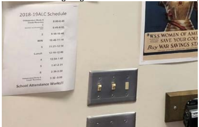
Photo 4: Basic Lighting Controls
