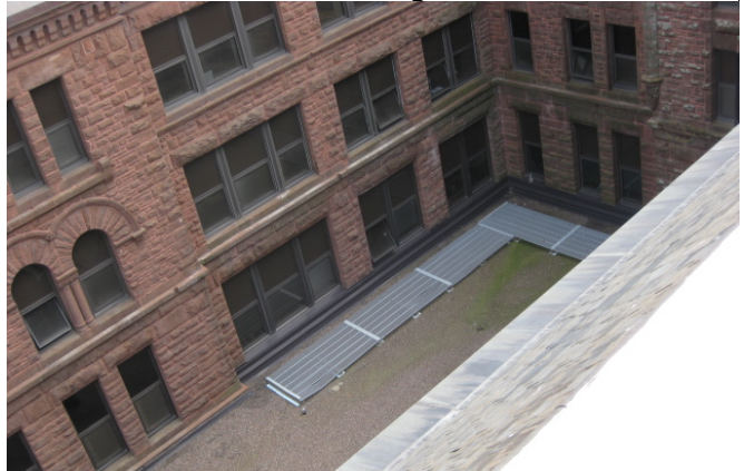
Photo 6: Protection from falling snow and ice
