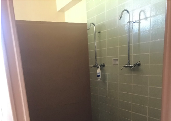
Photo 5 Showers do not comply with Code
