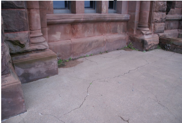
Photo 3: Cracked concrete landing
