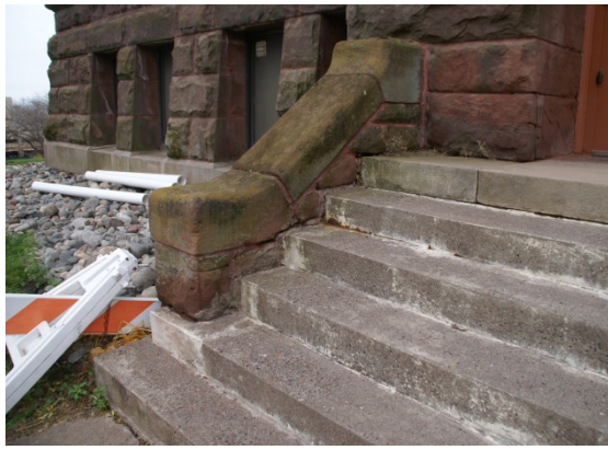
Photo 9: Deteriorated mortar and stone
