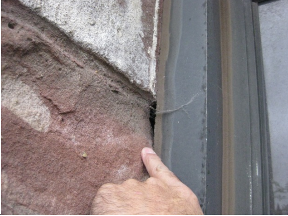
Photo 1: Open and deteriorated perimeter sealant
