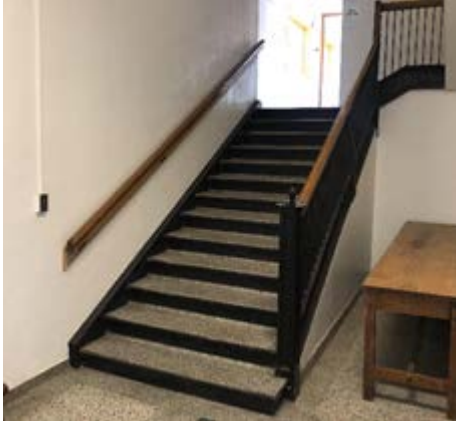
Photo 1 Accessible Route – No access to music room
