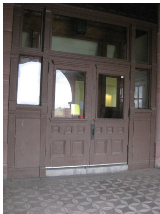
Photo 5: Poor condition main entrance doors
