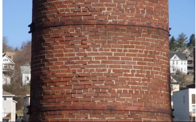
Photo 14: Deteriorated chimney masonry
