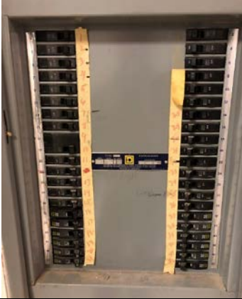
Photo 1: Full Electrical Panel
