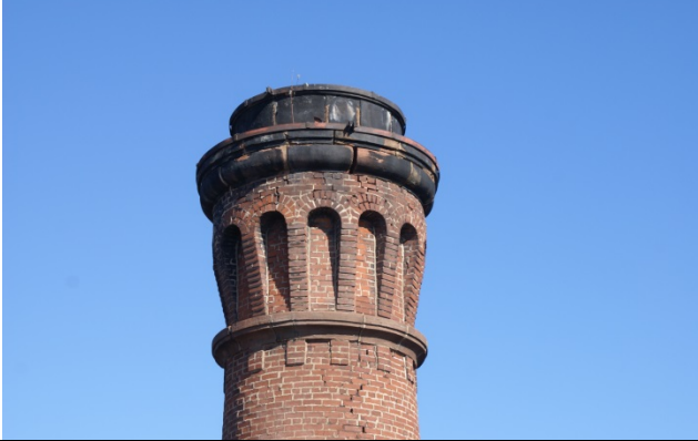
Photo 13: Deteriorated chimney cap
