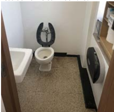
Photo 5 Restrooms – Clear Floor area
