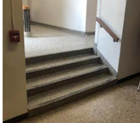
Photo 2 Accessible Route – No access to Men's room
