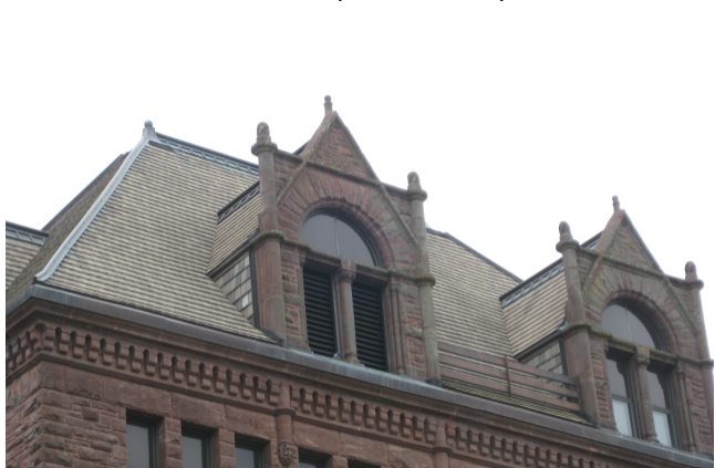
Photo 5: Snow retention (wood fence)
