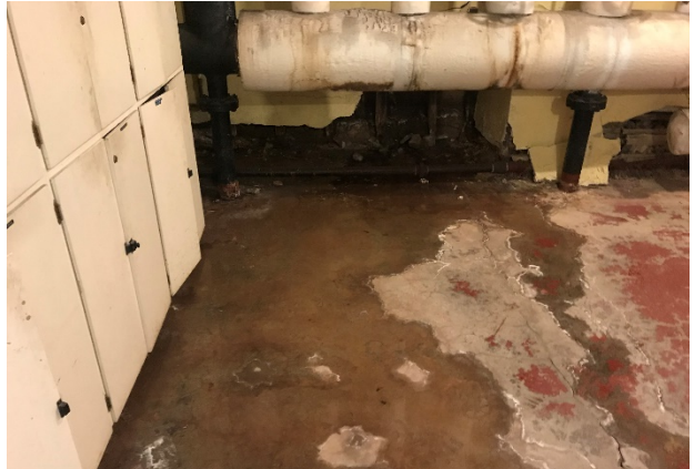
Photo 6 – Foundation Drain Failure
