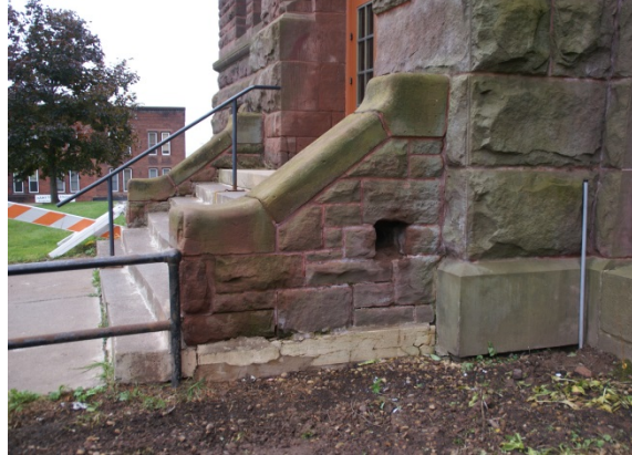
Photo 10: Deteriorated side wall
