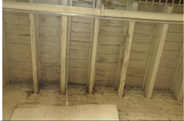
Photo 2: Sagging wood subfloor and joists
