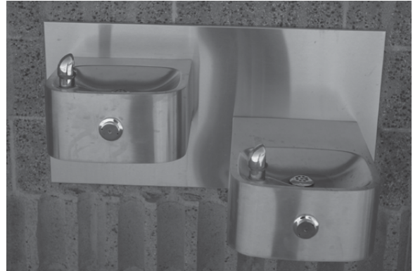
Fountains Connected to a Central Chiller
