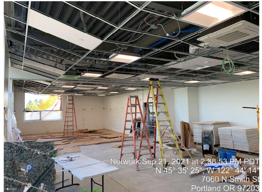
New classroom on 1 st floor of RHS P4 addition, will receive an operable partition wall.
