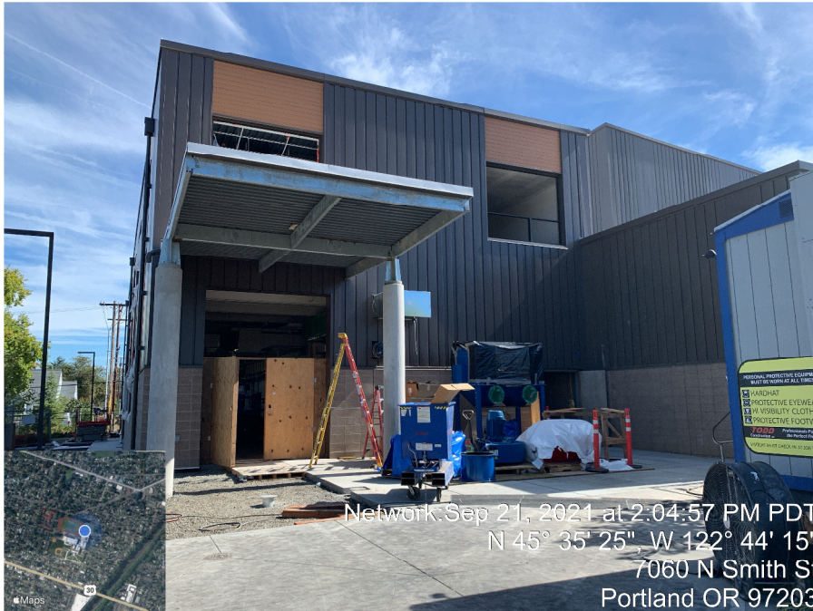
West side of RHS P4 addition showing CTE overhead door opening and dust collection equipment.
