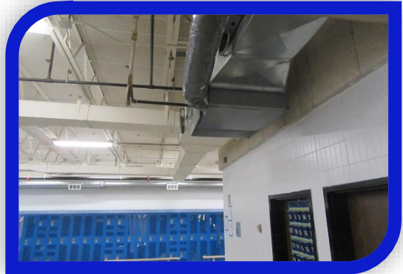
Locker Room Terminal Unit
