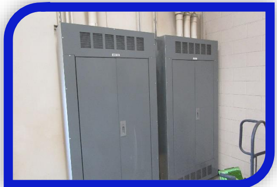
Main Electrical Distribution System
