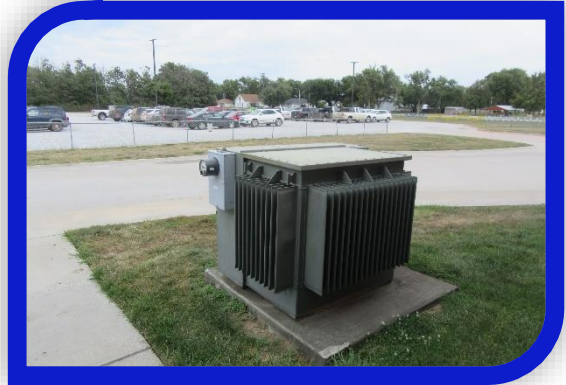
1 of 2 Transformers Serving Building
