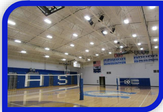
High Bay Lighting System
