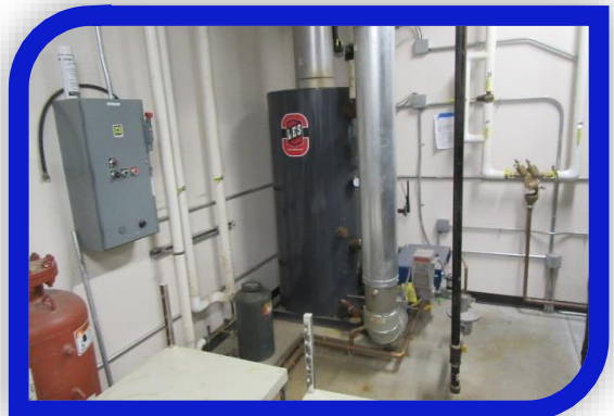
Hot Water Boiler
