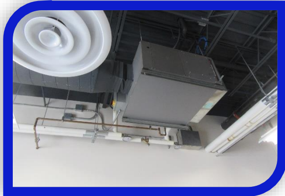
HVAC Terminal Unit
