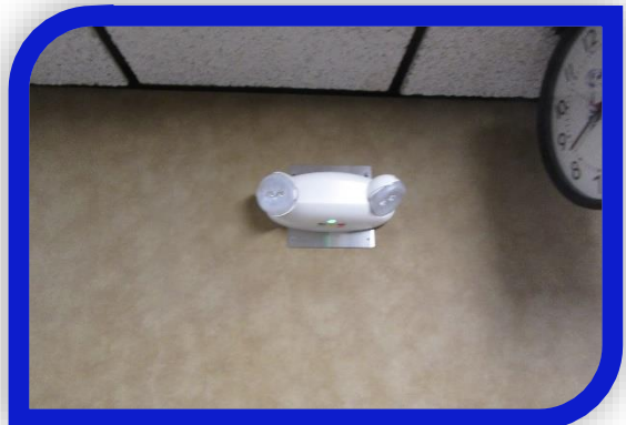
Emergency Lighting System
