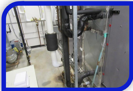
Air Handling Unit #1
