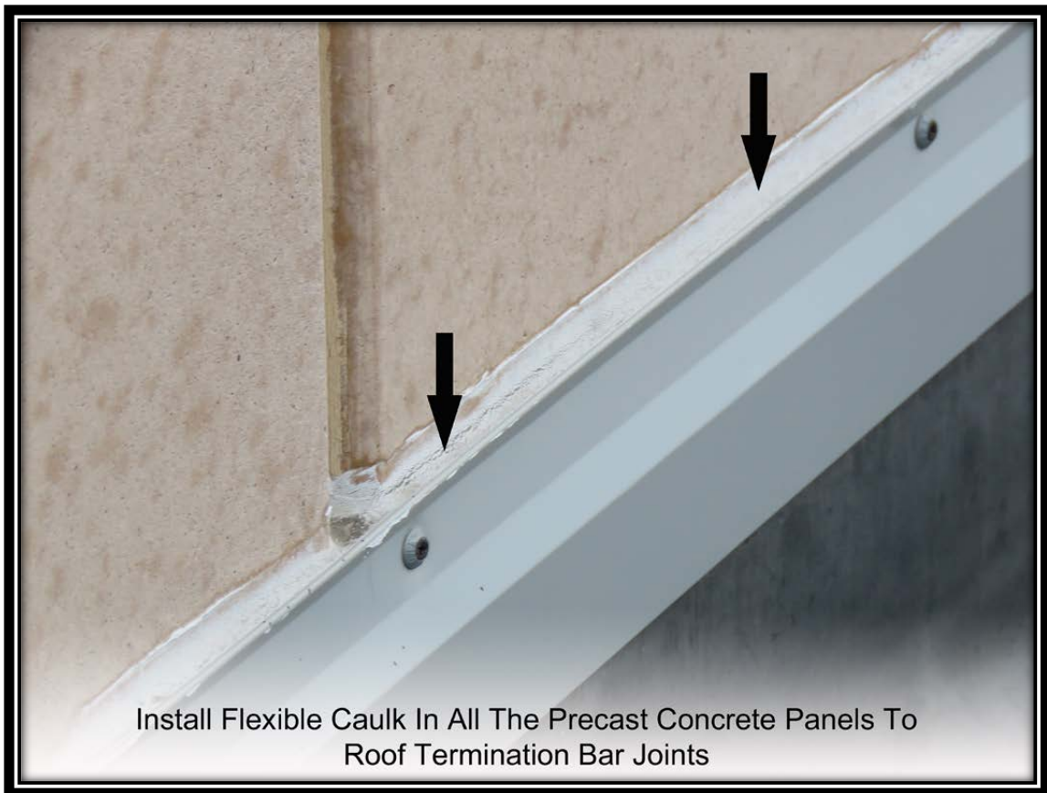
Install Flexible Caulk In All The Precast Concrete Panels To Roof Termination Bar Joints
