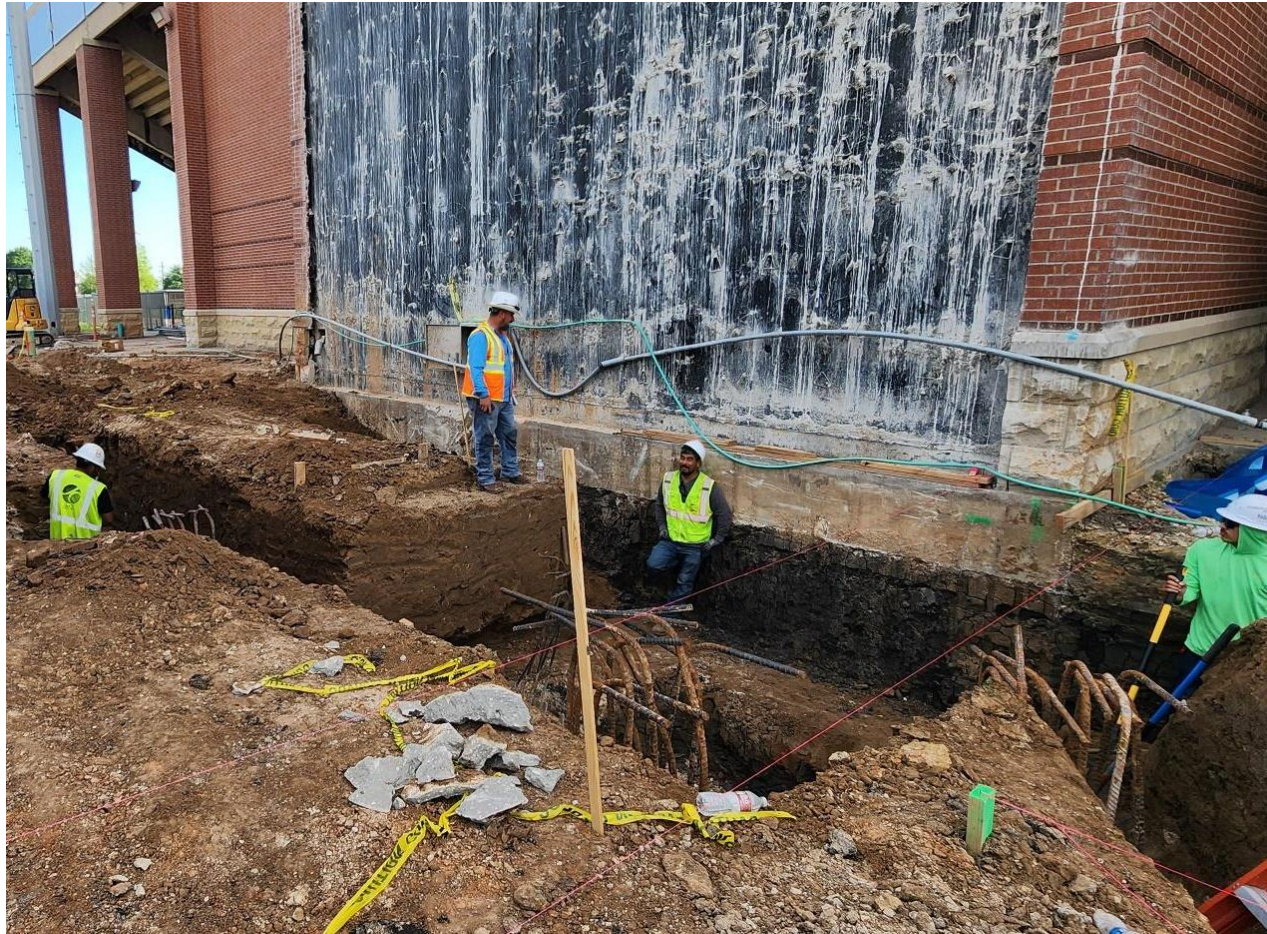
Concrete drilled piers have been placed, grade beam steel cage installation underway
