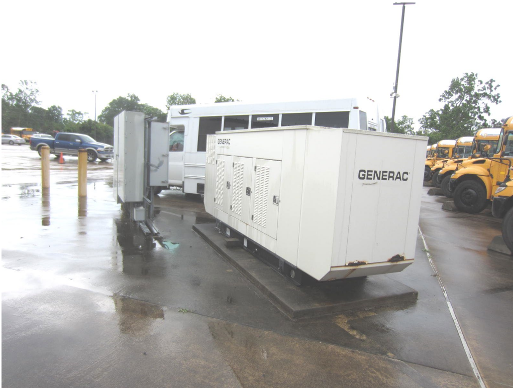
VIEW OF GENERATOR
