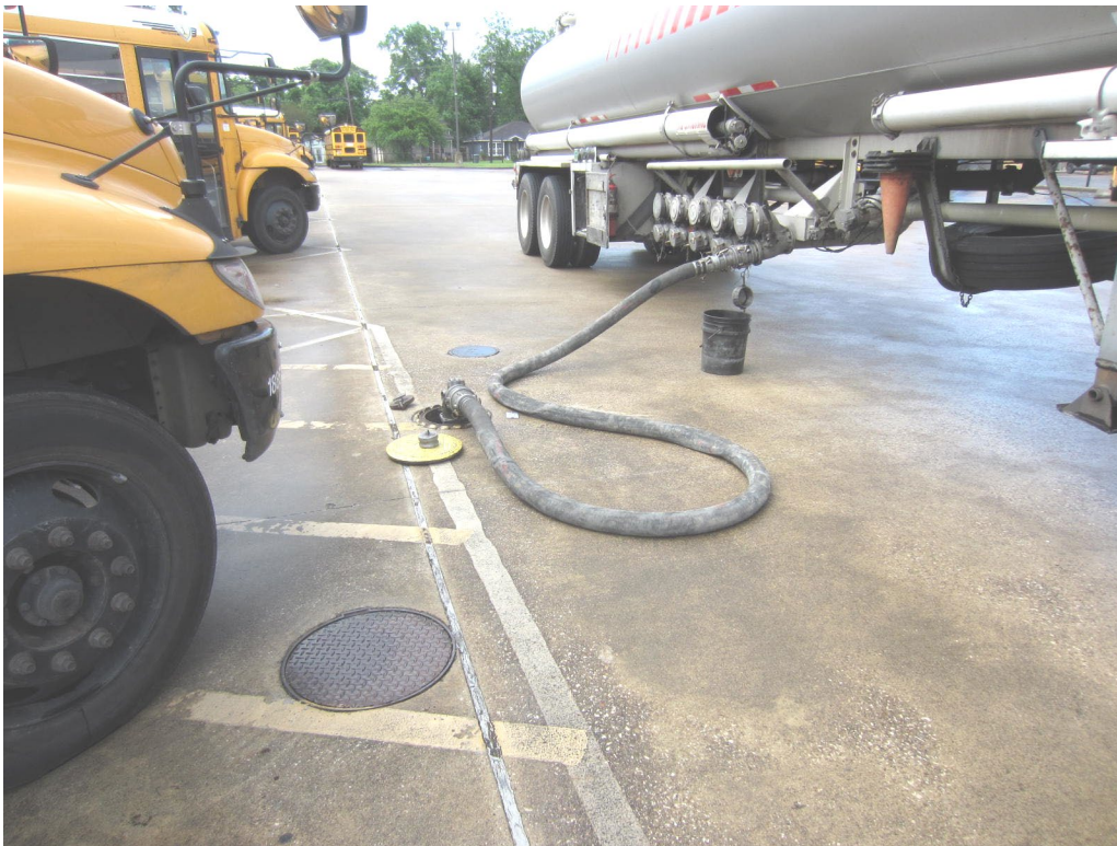
VIEW OF UNDERGROUND FUEL STORAGE TANK
