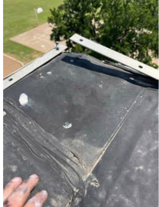
Term bar needs to be re-fastened
