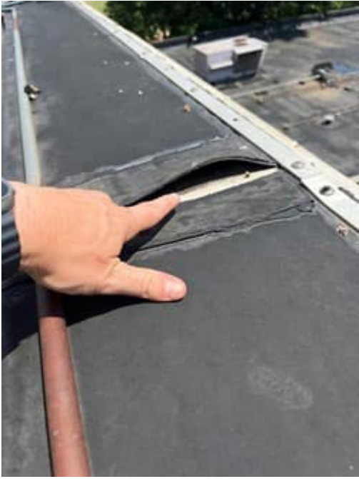
Open seam along coping
