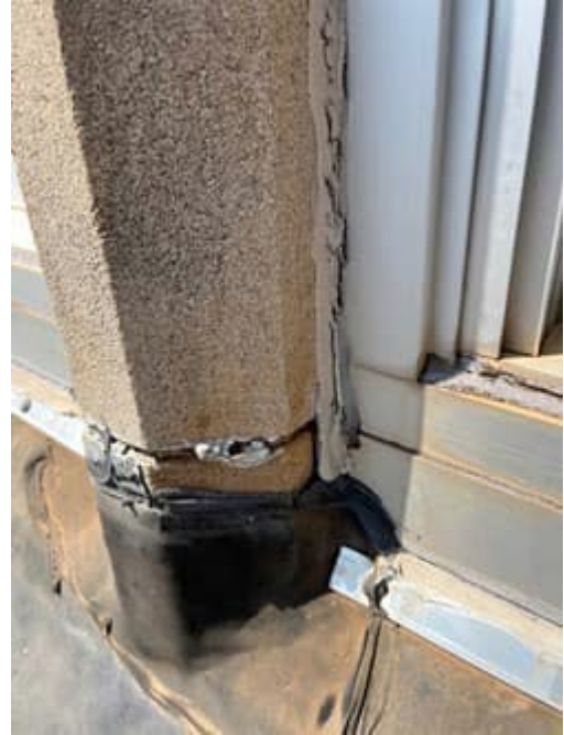
Masonry needs to be re-sealed
