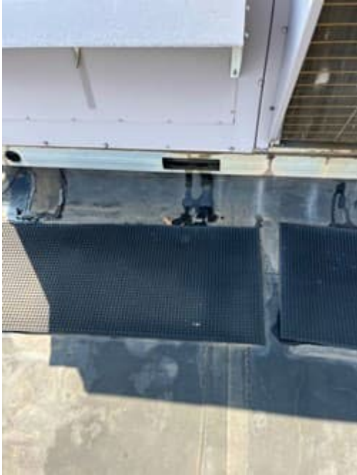
AC Unit is leaking
