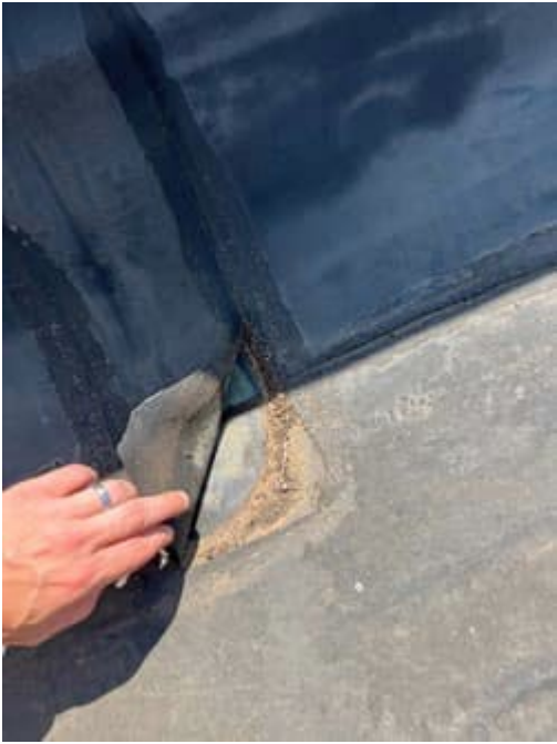
Exposed seam on parapet
