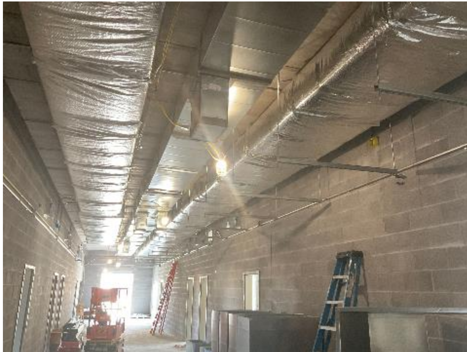
First Floor Corridor HVAC Ductwork
