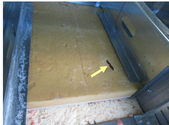
Figure 8. Roof fastener bent downward.
