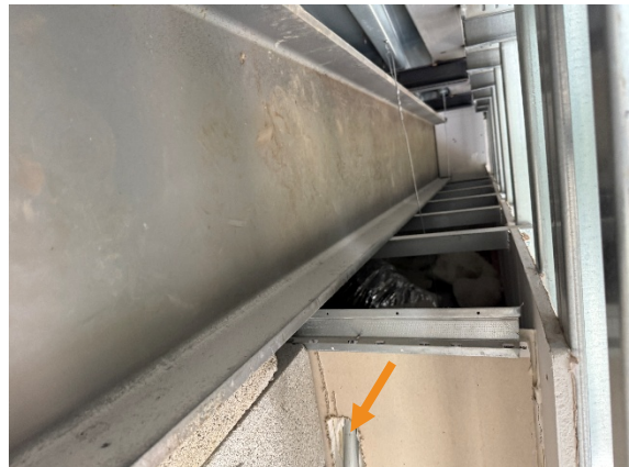
Figure 12. Top of interior wallboard at punched window jamb. Note the conduit at the top of the wallboard (arrow).
