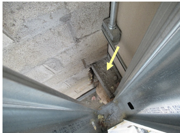
Figure 6. Gypsum wallboard to bear on concrete floor slab near base of wall (arrow).
