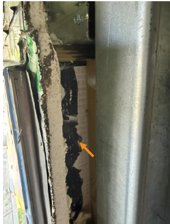
Figure 9. Punched window jamb with additional ArmorWall removed. At this location, there is an ArmorWall sheathing return at the jamb. Note the black material on the backside of the sheathing (arrow). Photo courtesy of Ward.
