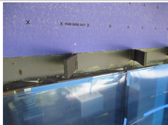
Figure 9. Window head condition at sunshades.
