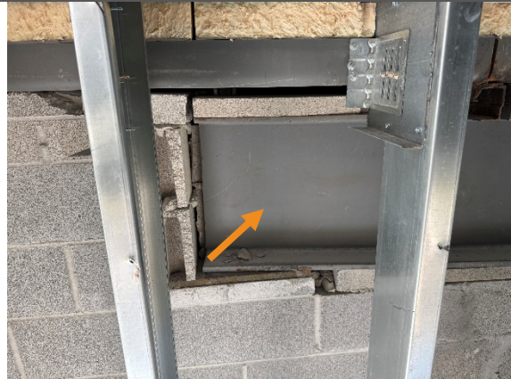
Figure 10. Beam bearing on CMU wall at north elevation. Note that the CMU is not continuous to the underside of the roof deck.
