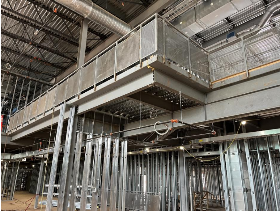
AREA 4 – STUDENT CENTER SECOND FLOOR RAILING
