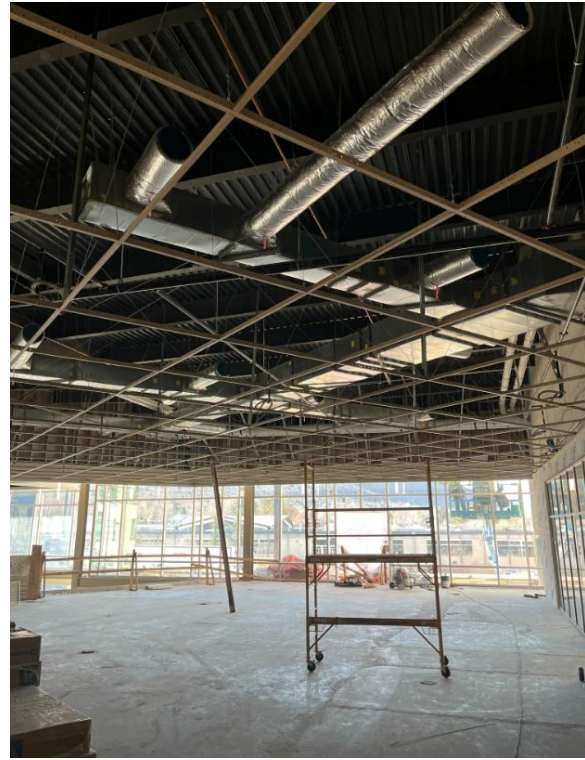
Wood-look acoustical ceiling grid outside of Level 2 Media Center
