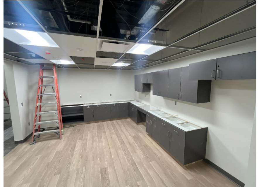
Cabinets installed in the Administration Suite Workroom
