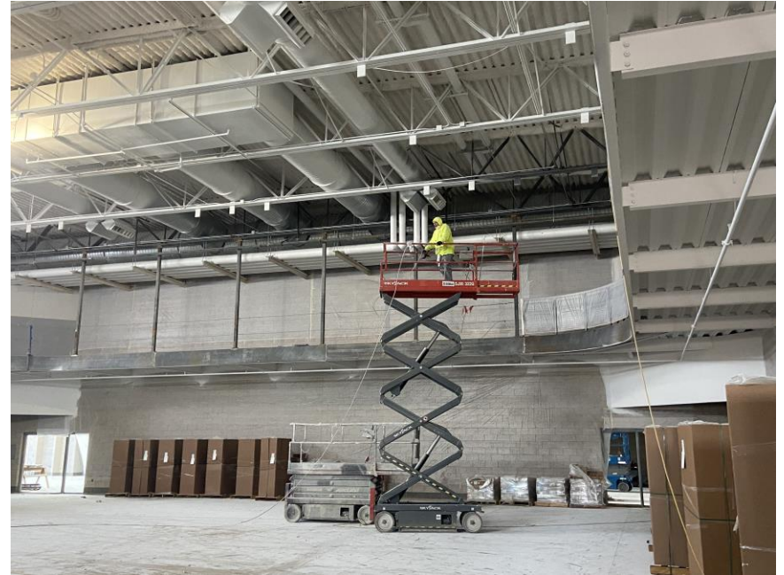
Ceiling paint in Gymnasium
