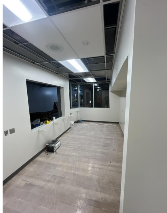
248 LVT flooring and glass installed in Fix-It Room by the Media Center on Level 2
