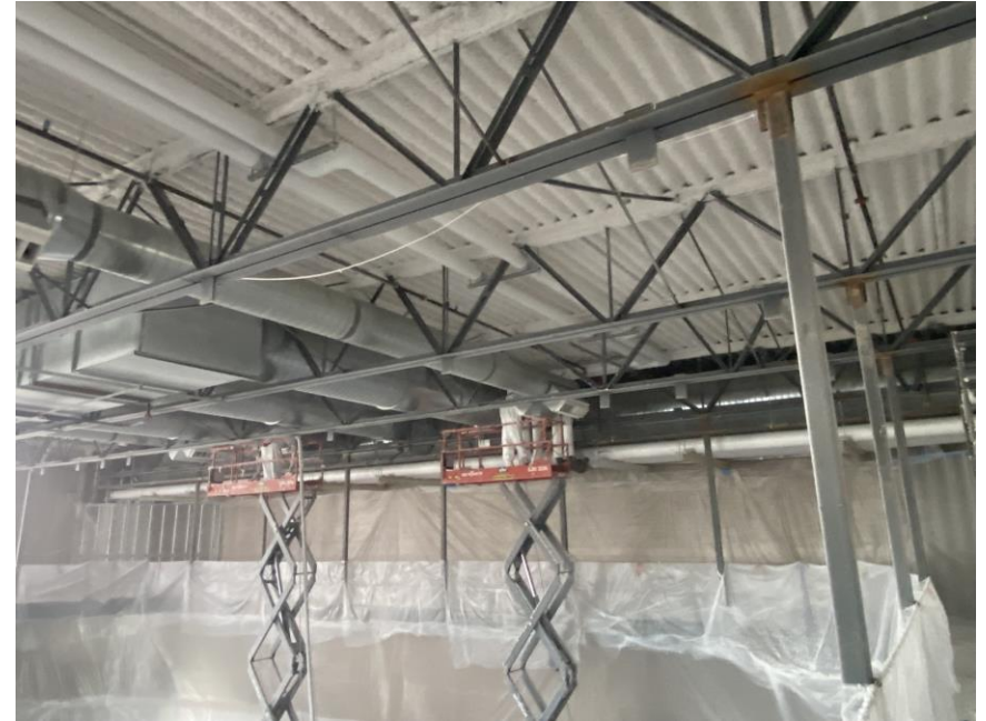
Acoustical treatment in Gymnasium
