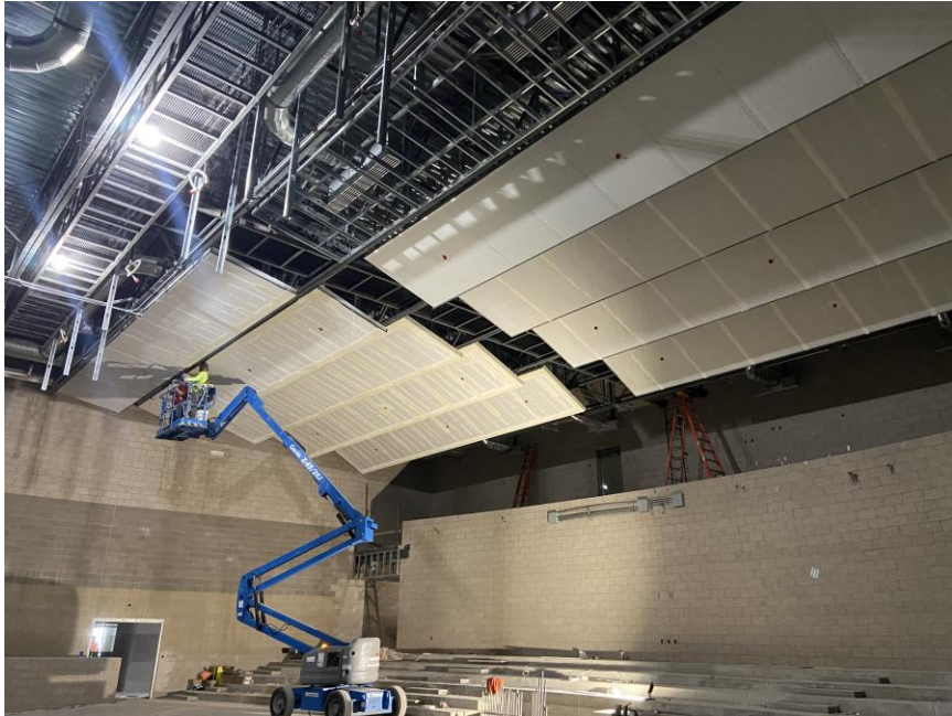
Sound panels in Auditorium
