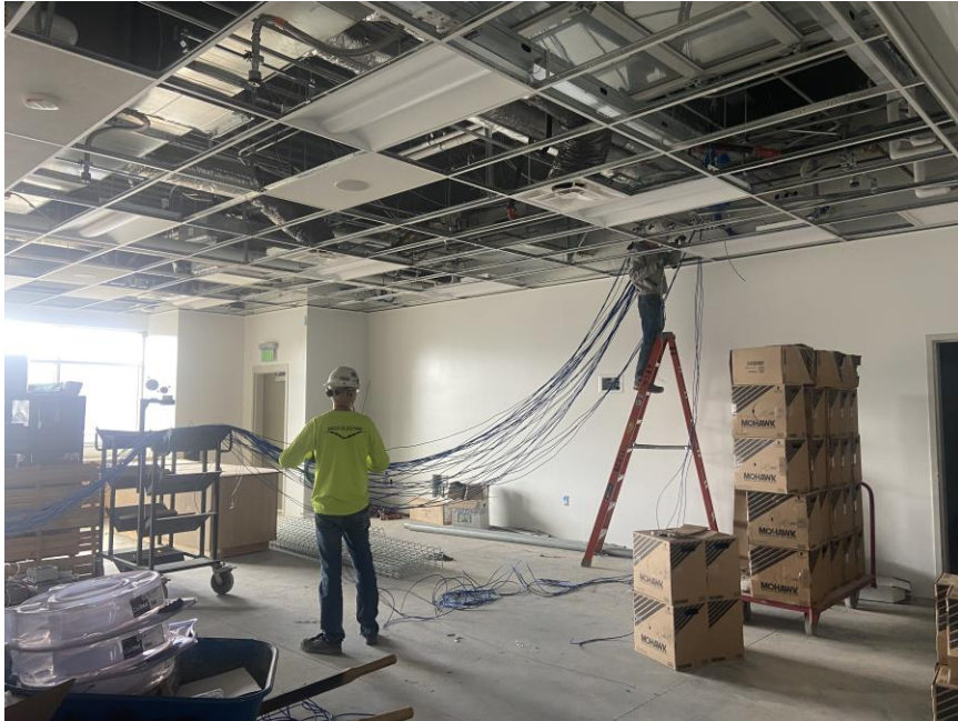
Communication wiring in classrooms
