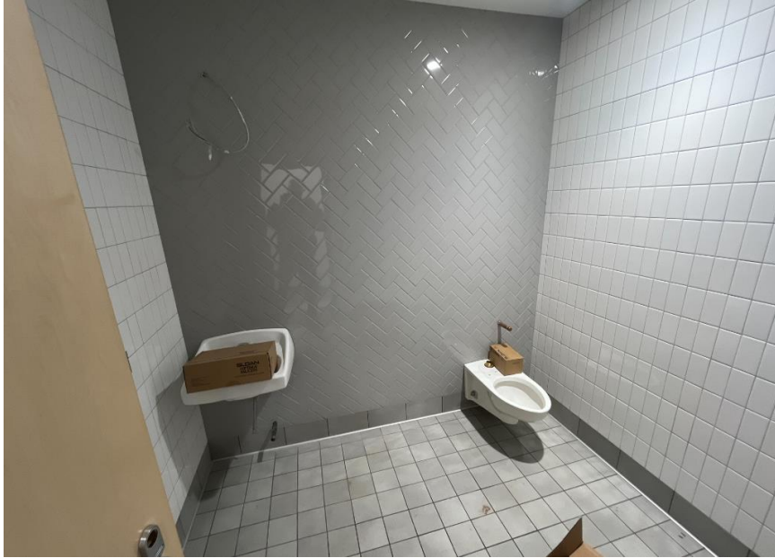
Plumbing fixtures in Administration bathrooms
