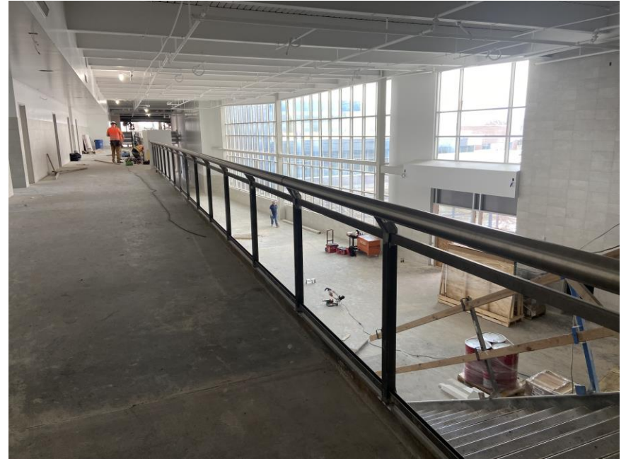
Railings in the Commons Area
