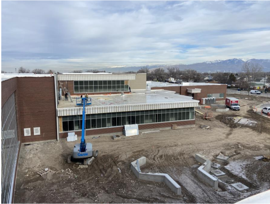
Insulation and decorative metal panels
