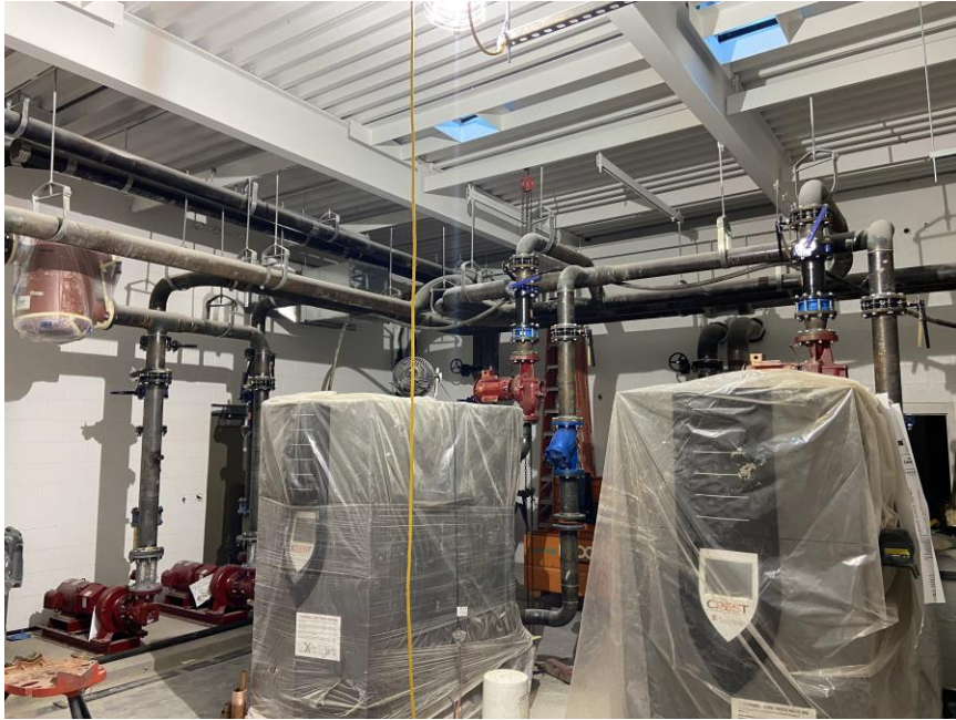
Pumps and piping in boiler room
