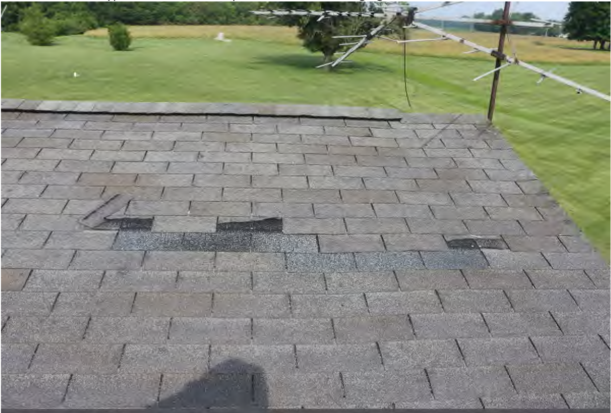
Photo No. C27: Torn, creased and detached shingle tabs on Maintenance Building roof.
