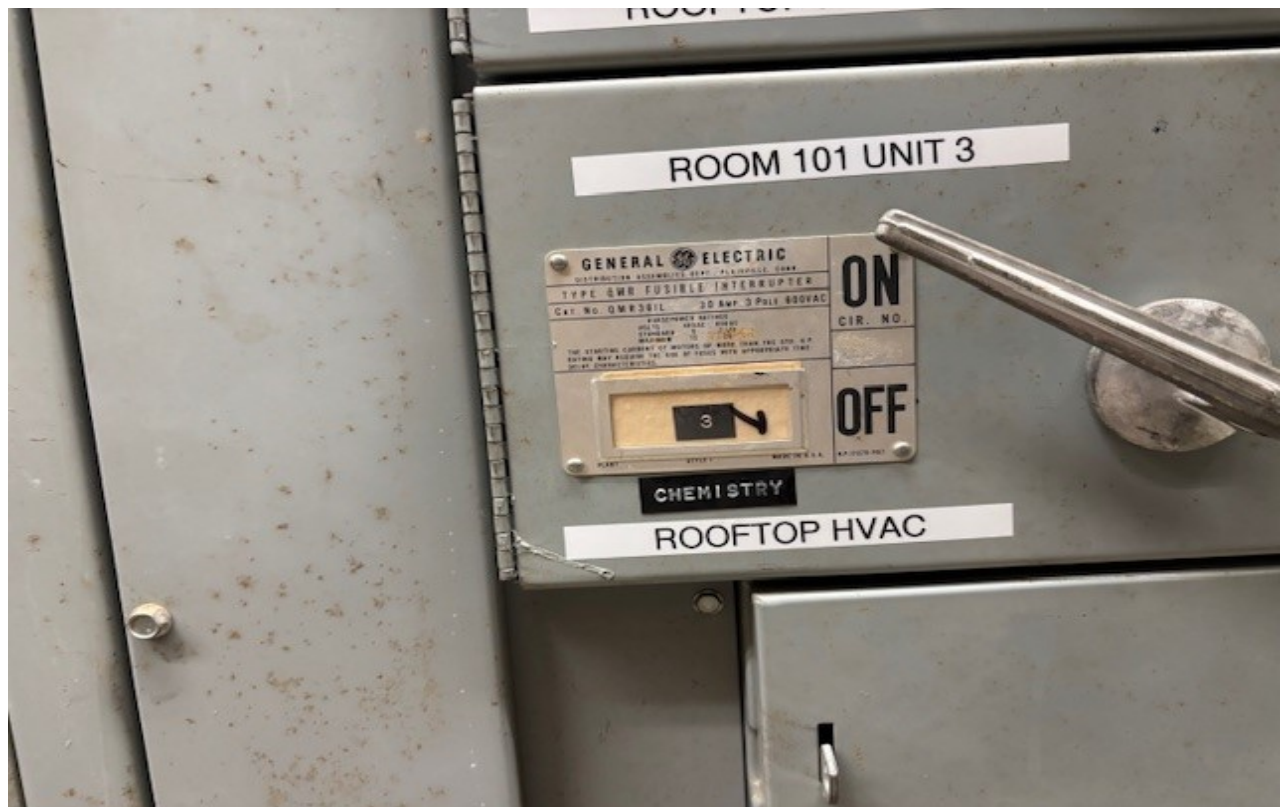
Electrical Panel Information
