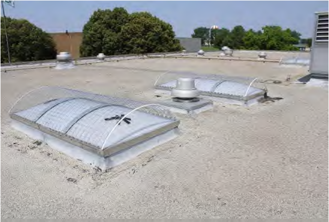
Photo No. B32: Skylight with two fractures on roof of Williams Hall
