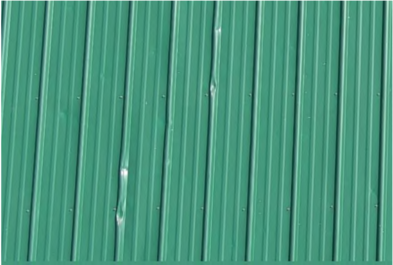
Photo No. B92: Enlarged view of dents/deformations at north-facing roof slope of LTC Foundation Pavilion – note disengaged seams
