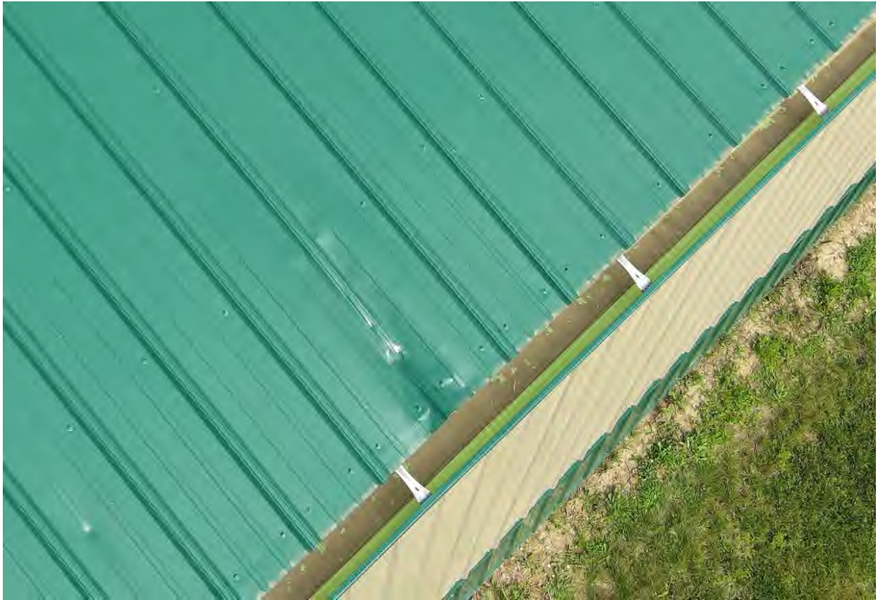
Photo No. C97: Indentations on the west-facing roof slope with disrupted paint coating.
