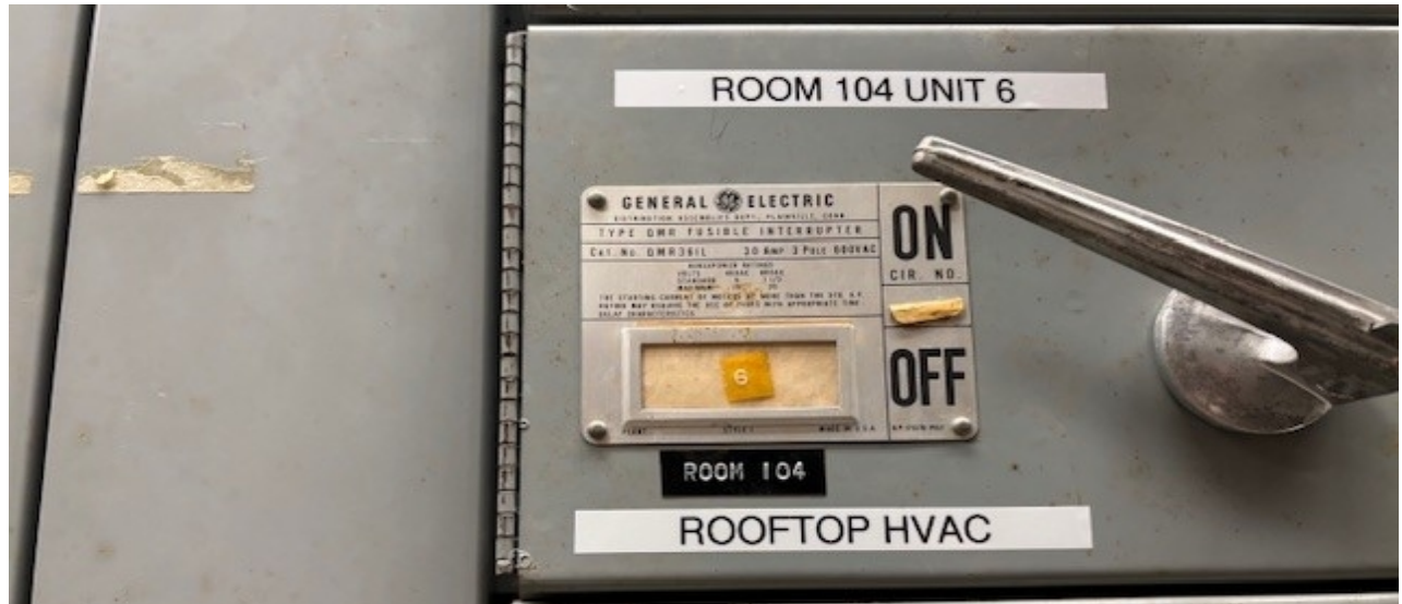
Electrical Panel Information
