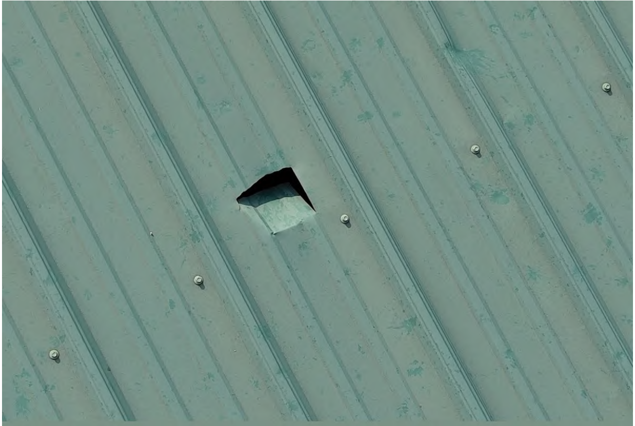
Photo No. C112: Detail of a punctured roof area, coincident spatter.
