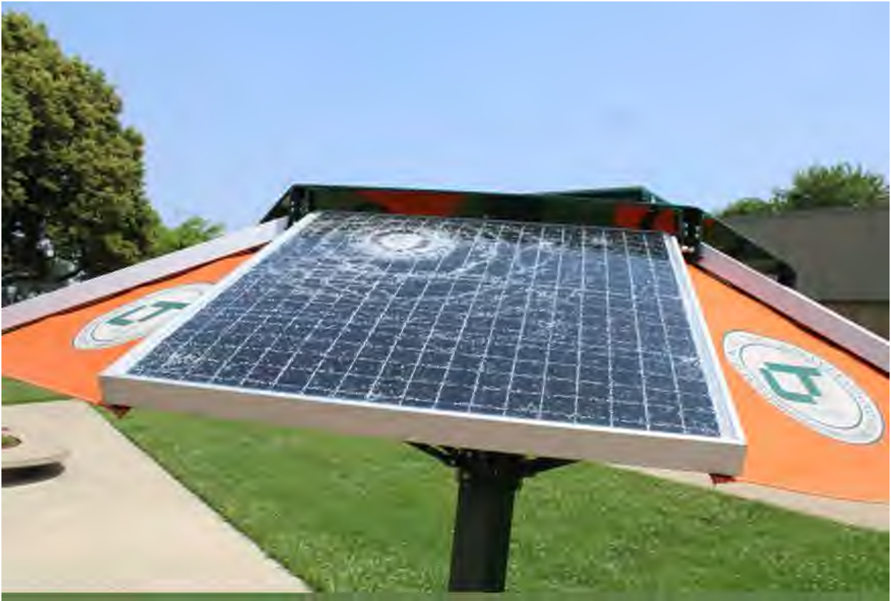
Photo No. B172: Typical fractured solar panel at outdoor charging station
