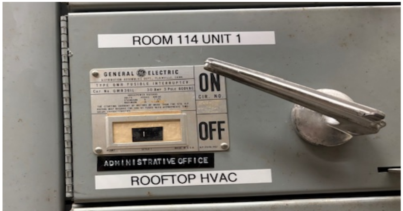
Electrical Panel Information
