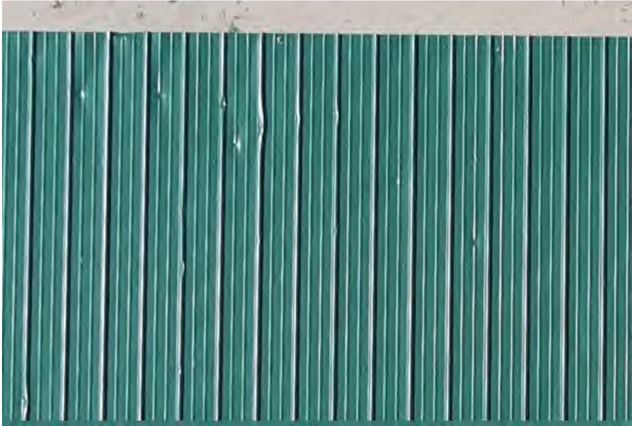
Photo No. B109: Enlarged view of dents at press box roof – note disengaged seams
