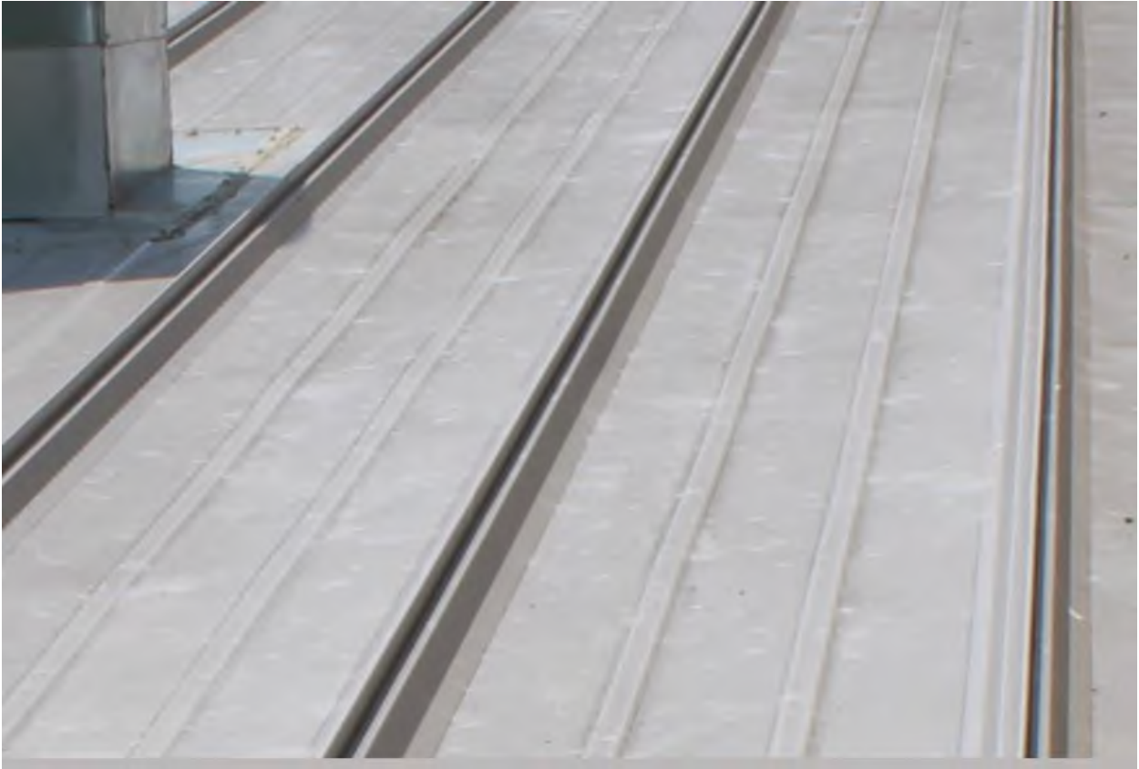
Photo No. B64: Enlarged view of dents in roof of Lackey Music Hall
