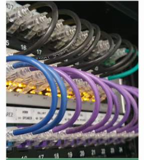
PATCH CABLES COLOR CODED & LABELLED
