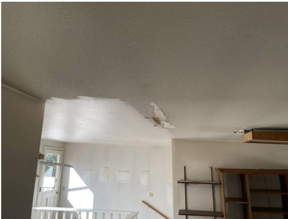
Figure 6- Damage to third floor ceiling.
