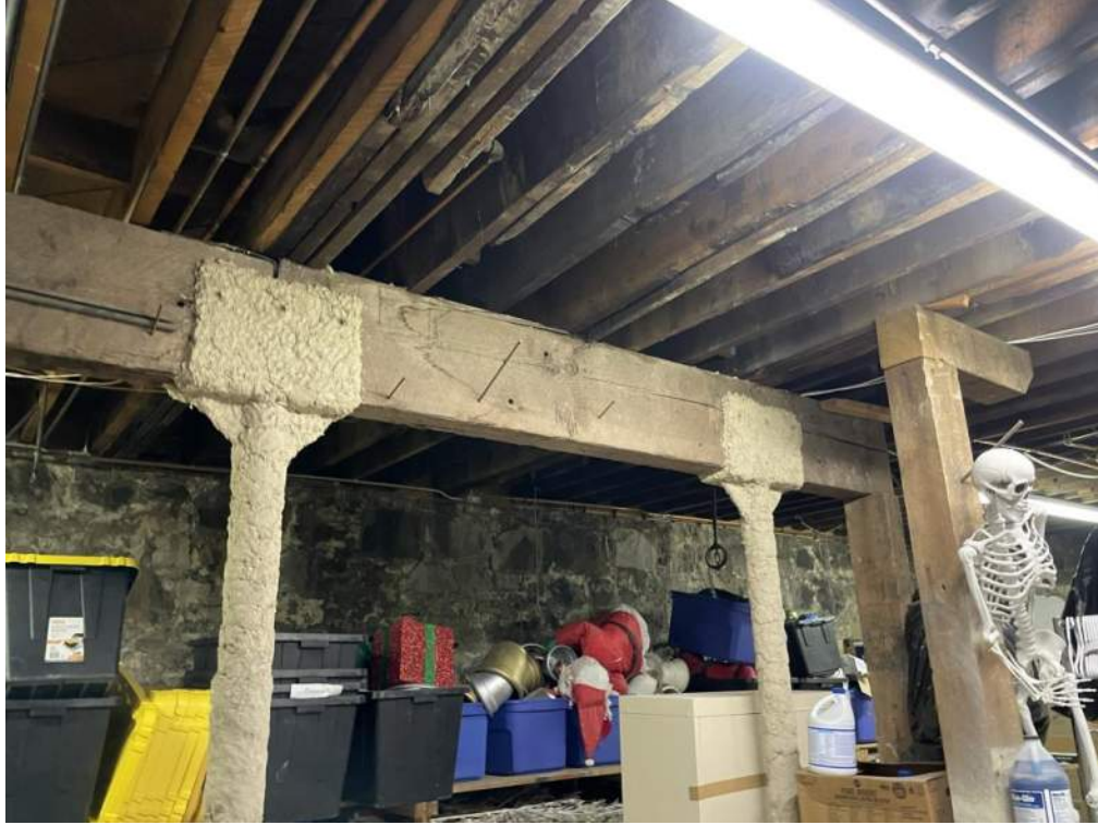
Figure 15- Upgraded framing in basement. Column locations correspond to hallway bearing walls above.
