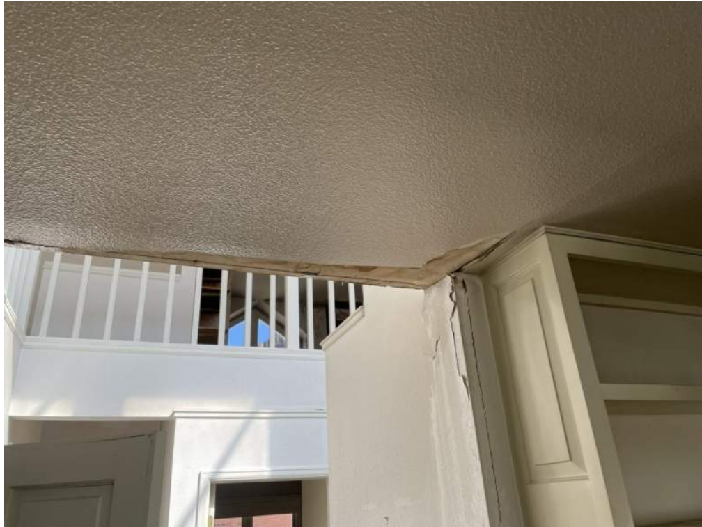
Figure 3- Damage to third floor framing at rear wall as viewed from the kitchen.
