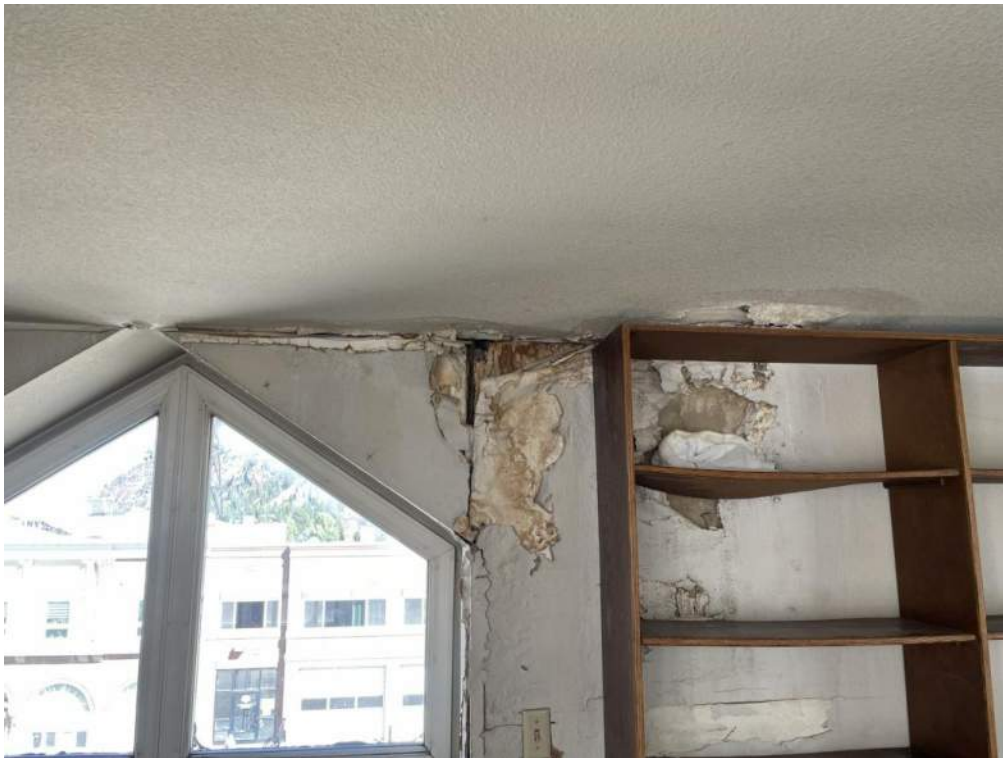
Figure 8- Damage at third floor bay window.
