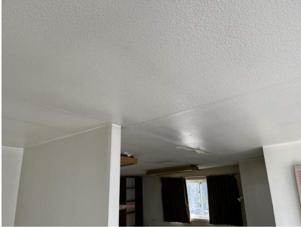
Figure 5- Damage to third floor ceiling.
