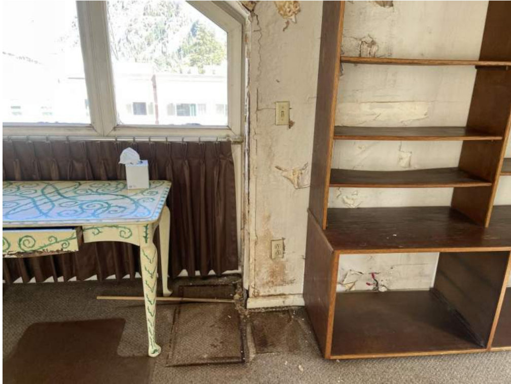
Figure 9- Damage at third floor bay window.
