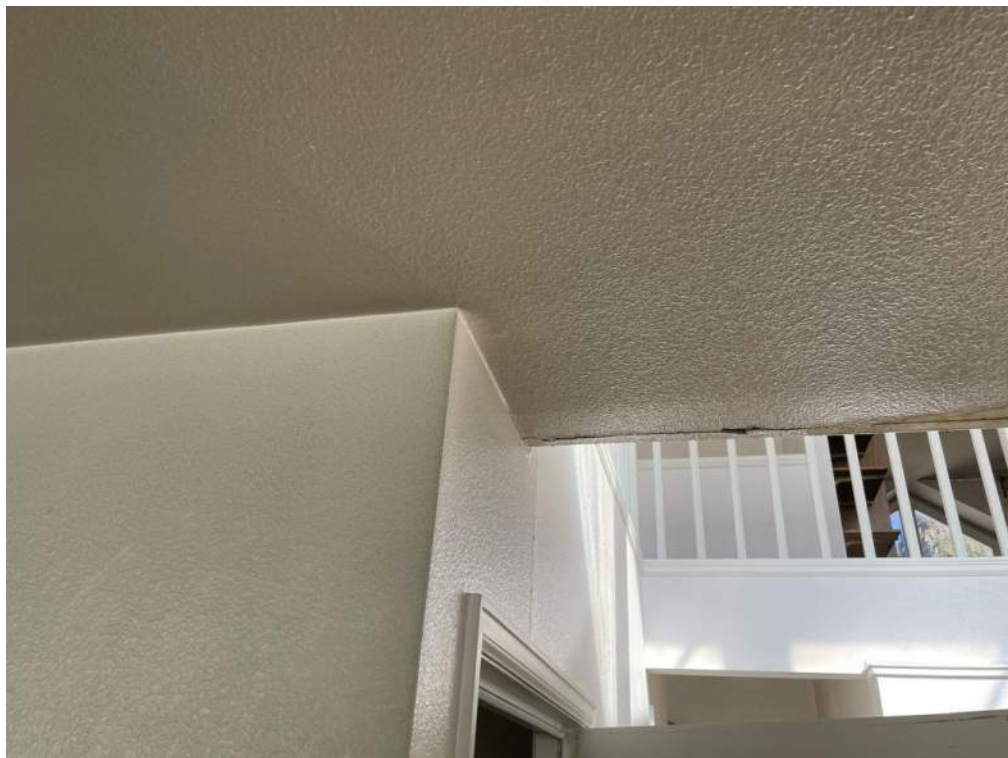
Figure 4- Damage to third floor framing at rear wall as viewed from the kitchen.
