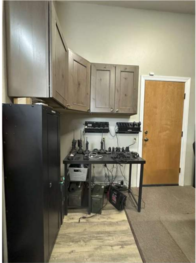
Supply area w/ mailboxes, in the open hallway area not ideal
