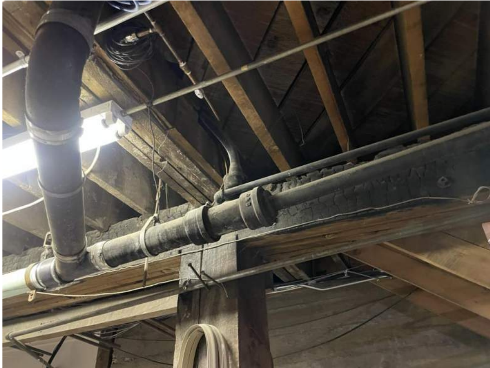
Figure 13- Example of main level framing in basement. Note charred beam and column.
