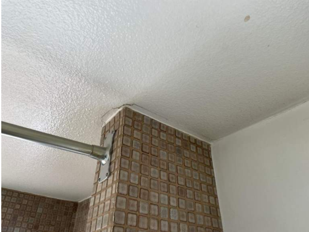
Figure 7- Damage to third floor ceiling.
