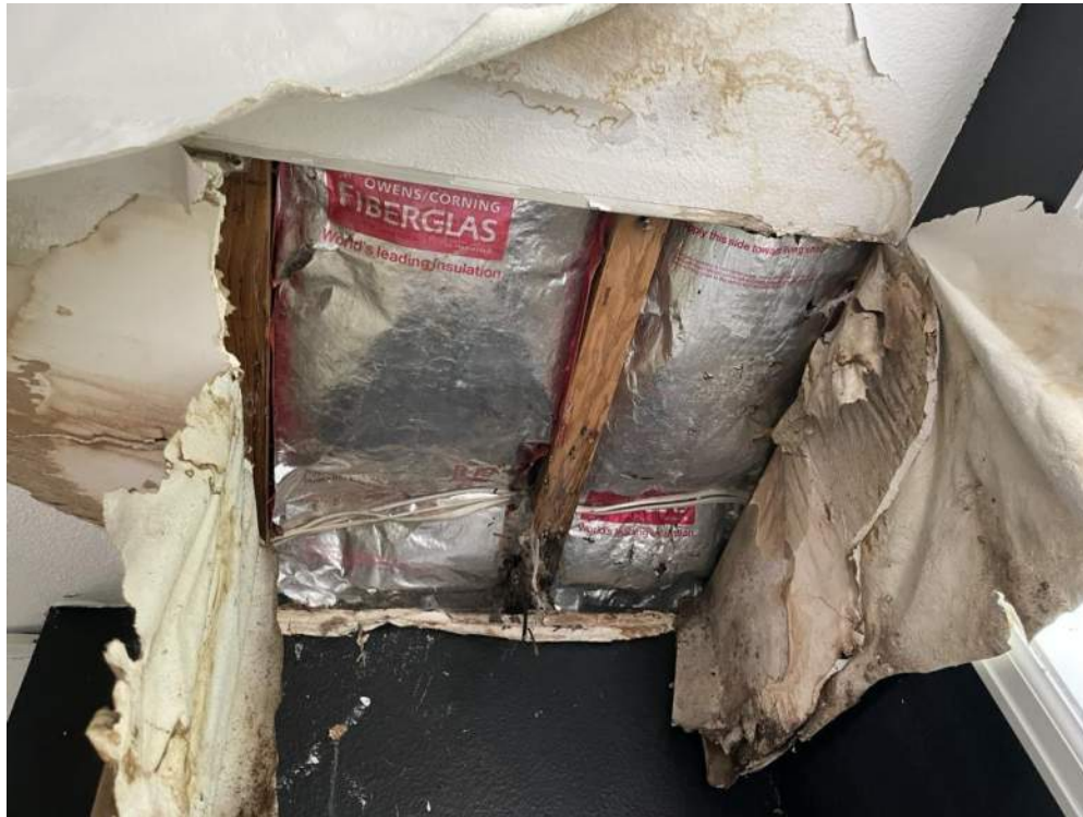
Figure 2- Exposed second level framing and evidence of water damage.
