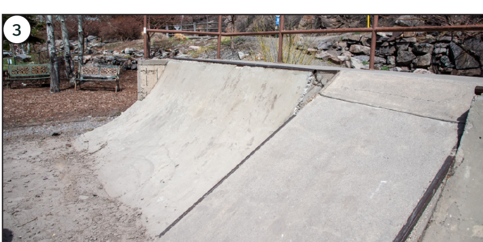
3 Skate Park Analysis: Deteriorating concrete needs improvement and or replacement.
