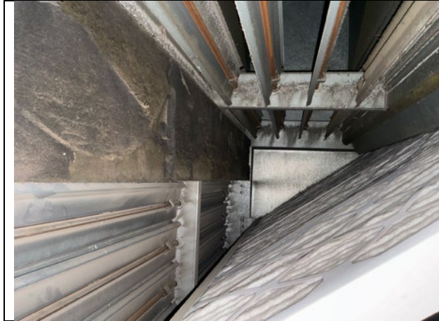
Outdoor air damper (top) is open Return air damper (left) is closed
