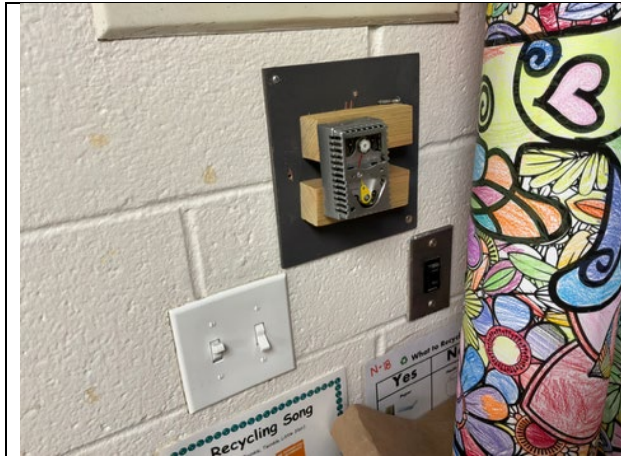
Pneumatic control of heating valve in unit
