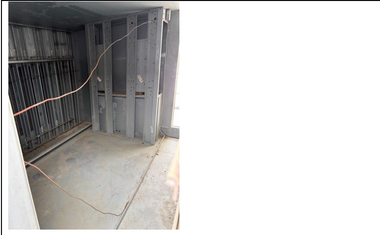
Mixed air temperature sensor
