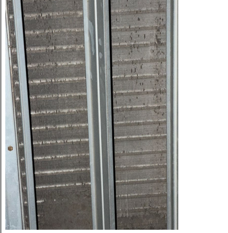
Dirty coil face inlet
