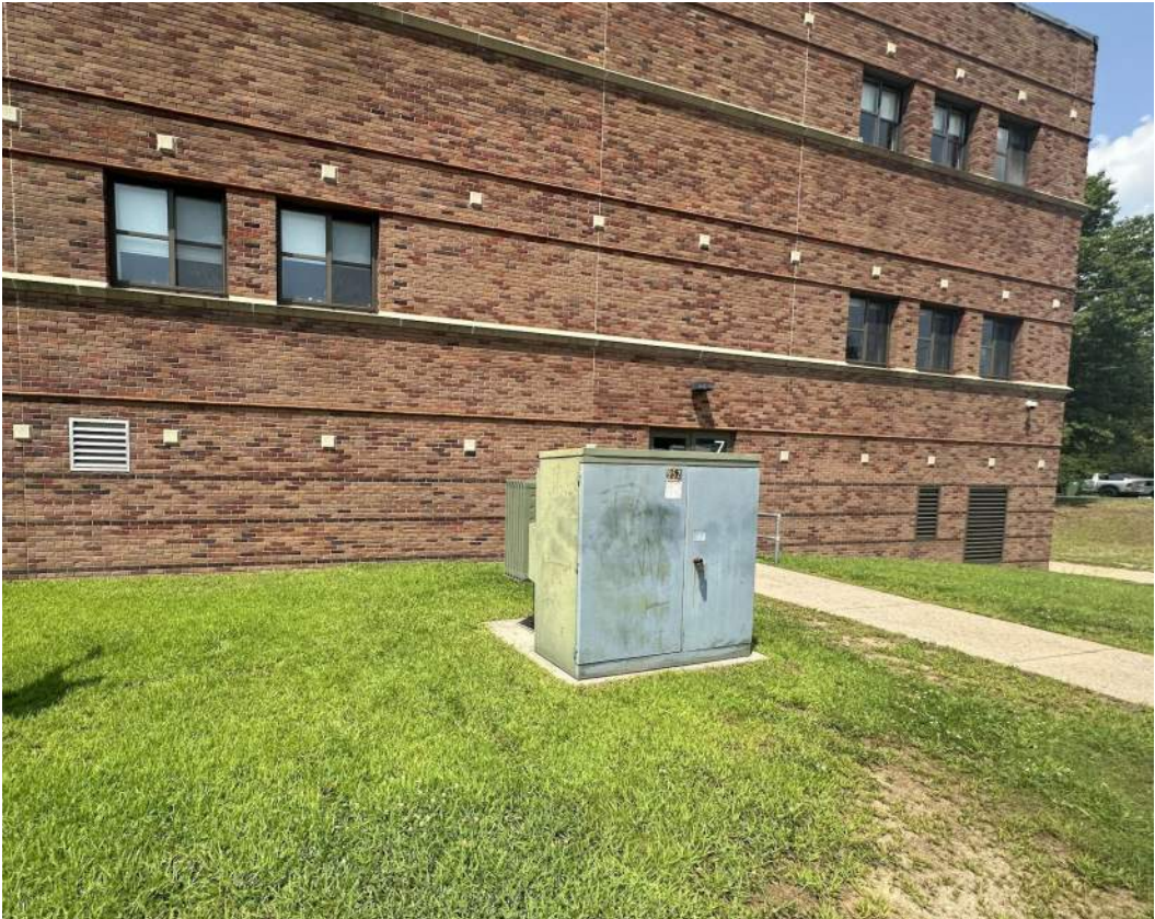
Exhibit 6: Photos of the existing utility transformer
