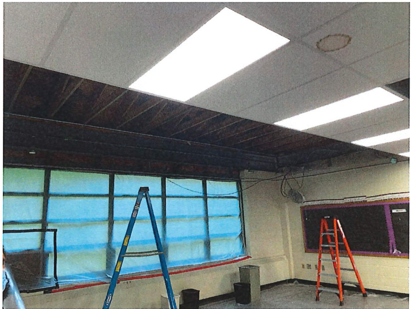
Snow School roof damages ^
