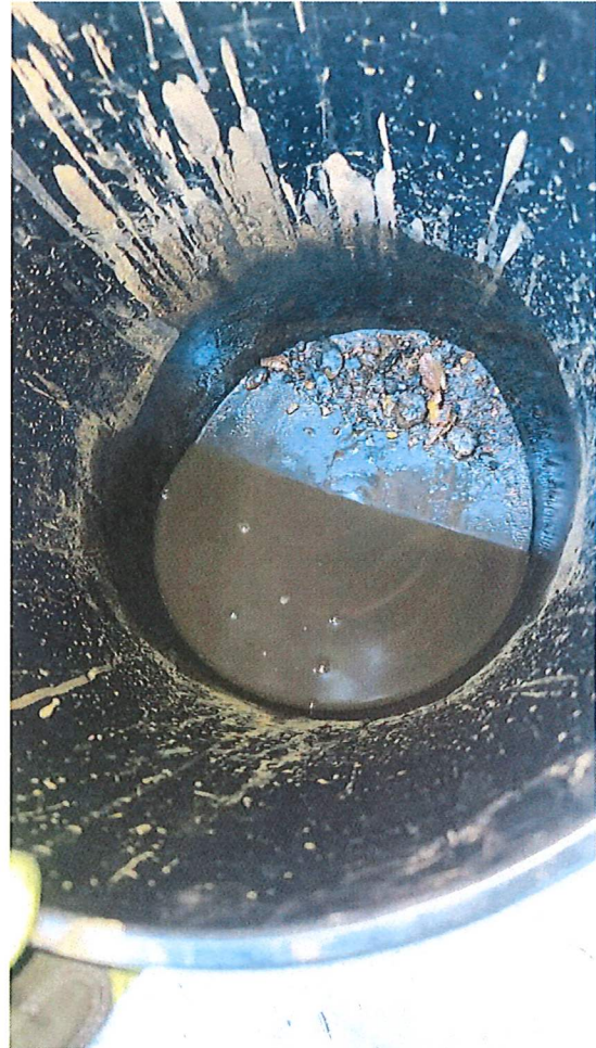
Adult Education fire sprinkler dry system ^
