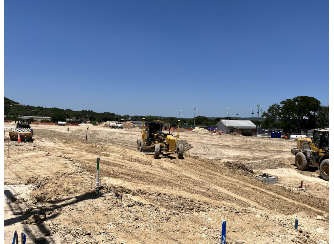
Photo: Utilities/Pad at Performing Arts
