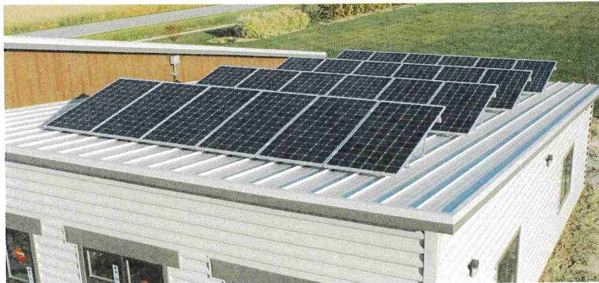
Example of a Solar Conversion System, Structure-Mounted
